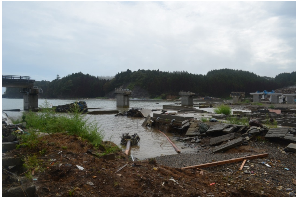
Figure 1. Utatsu Bridge failure during 2011 Great East Japan Earthquake and the subsequent Tohoku Tsunami (Photo by Yim).
