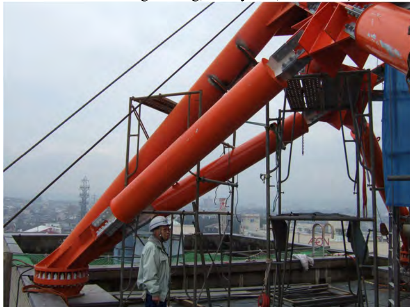
Figure A-31 Close Look of BRBs Installed in the Communication Tower (Courtesy of Ian Aiken, Seismic Isolation Engineering, Emeryville, California)
