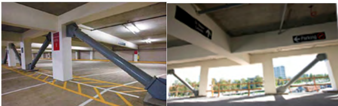
Figure A-32 Configuration of BRBs in Parking Building of John Wayne Airport ( http://www.airportimprovement.com/content/story.php?article=00258 )
