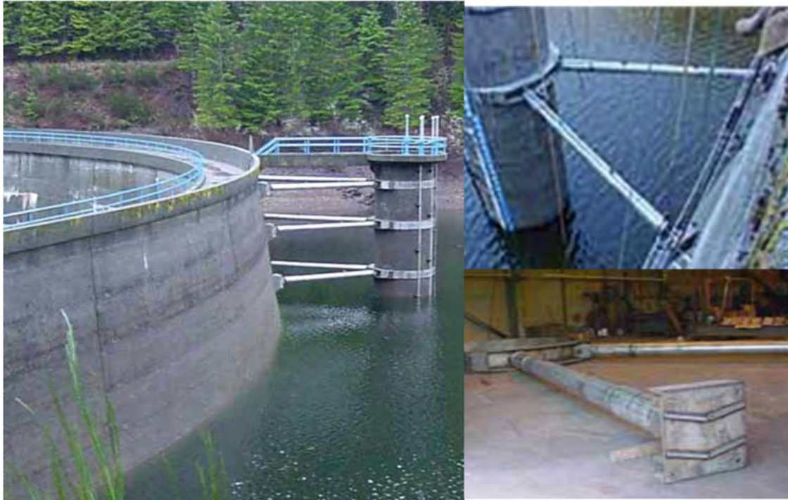
Figure A-33 BRBs Installed in Casad Dam ( http://www.starseismic.net/projects.html )
