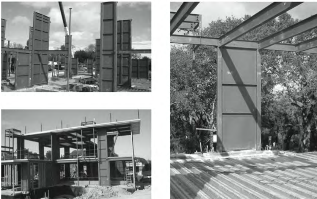
Figure A-62 Residential Building With SPSW In San Mateo County, CA (Sabelli & Bruneau, 2007)
