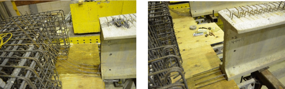
Figure 4.14: ESBF connection (left) prior to cutting one strand and inserting strands into cap beam; ESSP connection (right) prior to cutting one strand and attaching anchor plates and chucks
