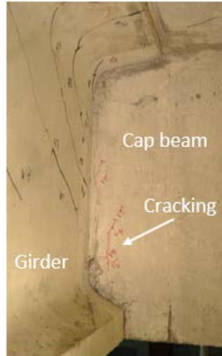
Figure 4.40: Cracking on side of cap next to girder interface
