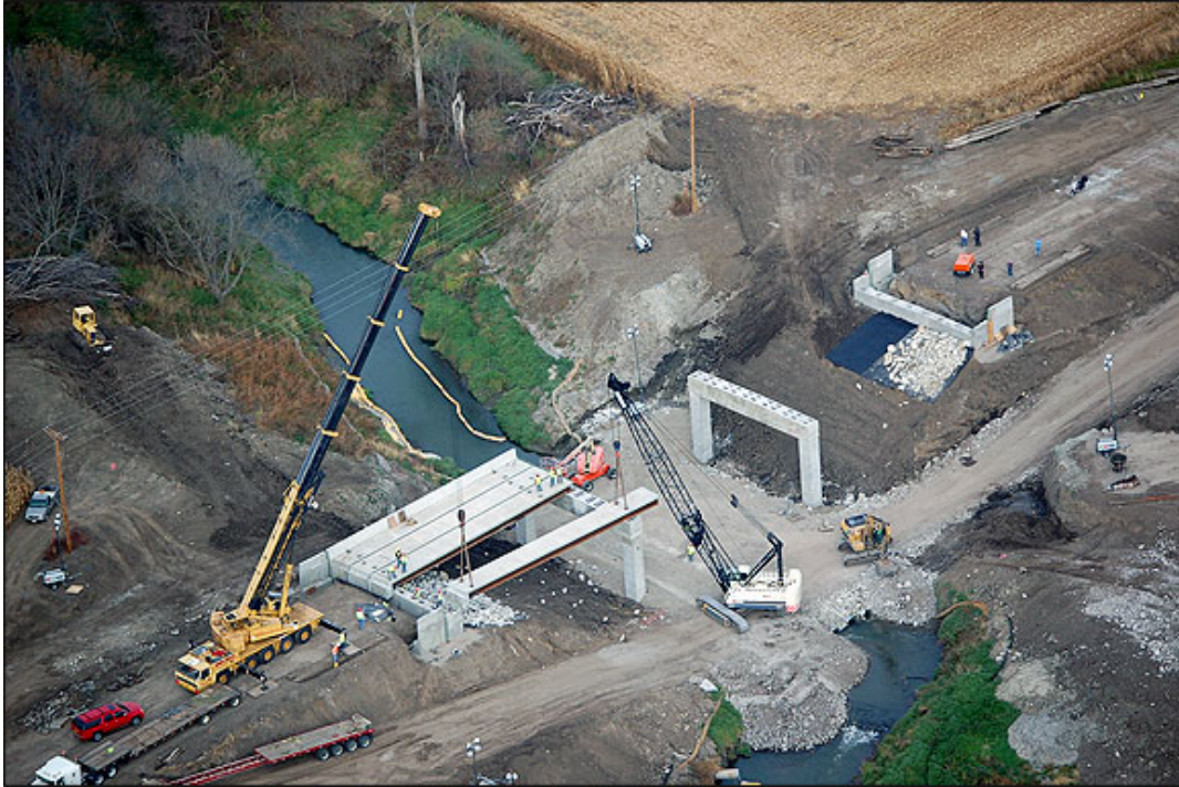
Figure 1.1: Keg Creek Bridge constructed using ABC methods (AASHTO, US 6 Keg Creek Bridge, 2011)
