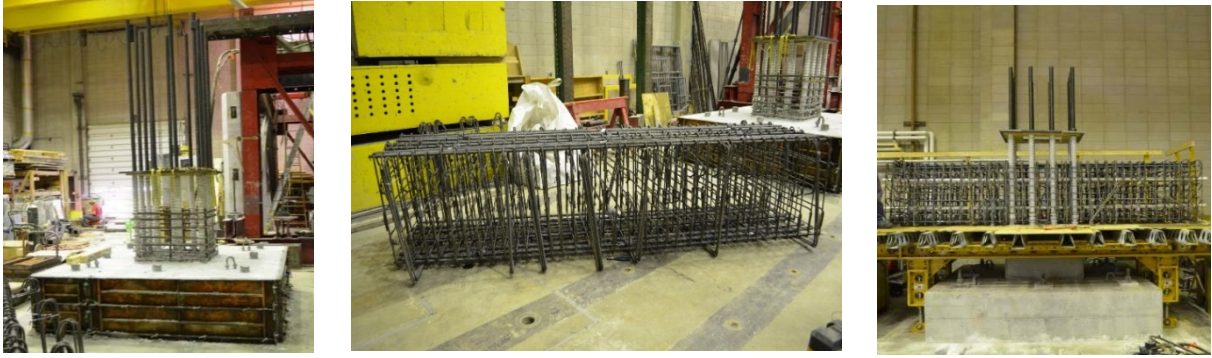
Figure 4.12: Footing and column pour (left); cap beam reinforcement cage (center); cap beam on platform (right)
