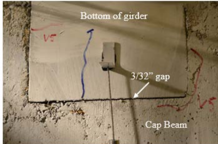
Figure 6.10: Gap observed between cap beam and bottom of girder
