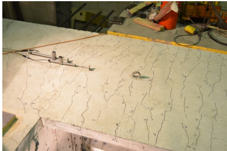
Figure 4.39: Girder cracking due to negative moment
