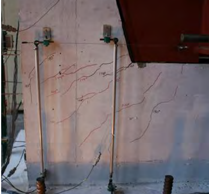
Figure 6.88 Crack behind the horizontal shear reinforcement of the stem wall on the west face of shear key 10A
