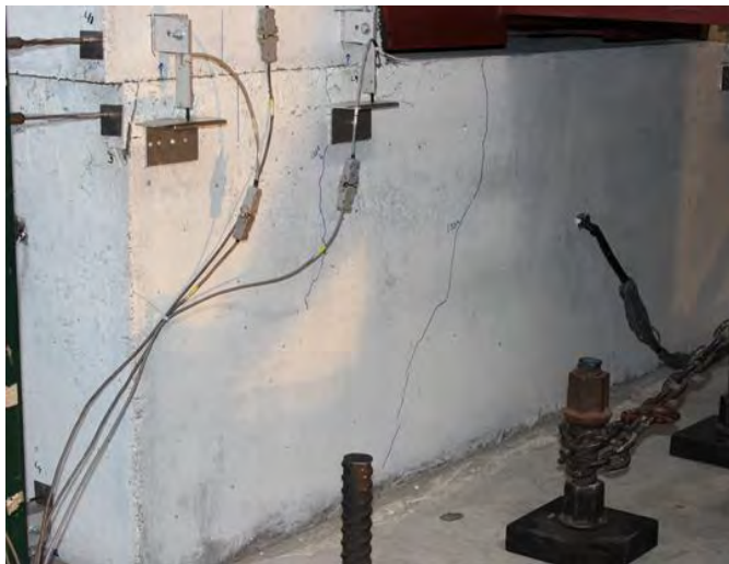
Figure 5.24 First two cracks observed on the east face of shear key 7A
