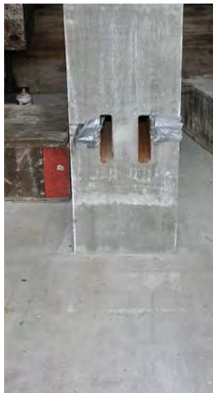
Figure 7.38 Stem wall and footing after shear key block was removed in Test 5
