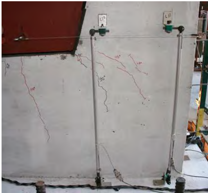
Figure 6.58 Propagation of first diagonal crack and additional cracks on the east face of shear key 9A
