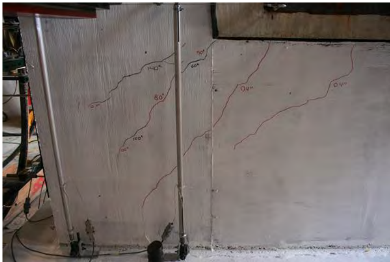
Figure 6.101 Cracks on the east face of shear key 10B at 190 kips
