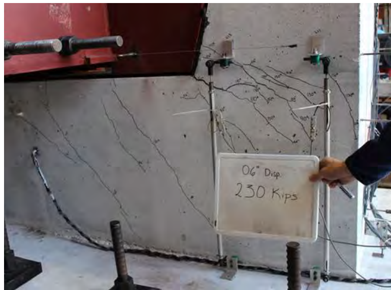
Figure 6.33 Cracks on the east face of shear key 8A at 230-kip load
