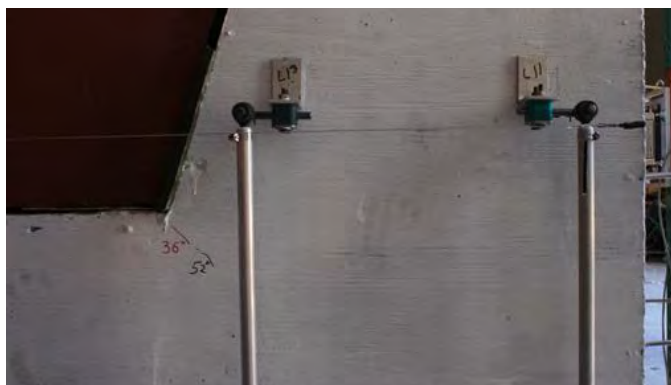
Figure 6.85 First diagonal crack observed on the east face of shear key 10A
