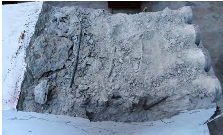
Figure 6.36 Sliding surface on stem wall after removing shear key 8A
