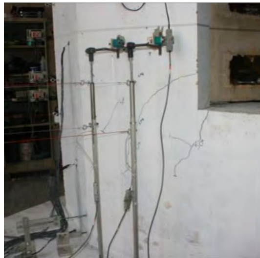
Figure 8.17 First cracks observed on the northwest side of shear key 12A
