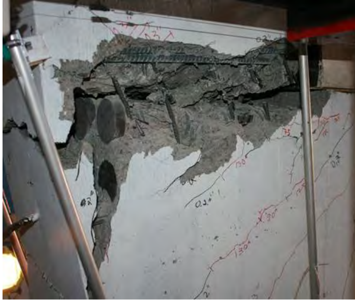
Figure 6.75 Fractured bars near the east face of shear key 9B
