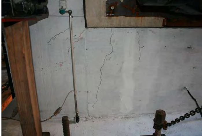
Figure 6.72 Propagation of first diagonal crack and additional cracks on the east face of shear key 9B
