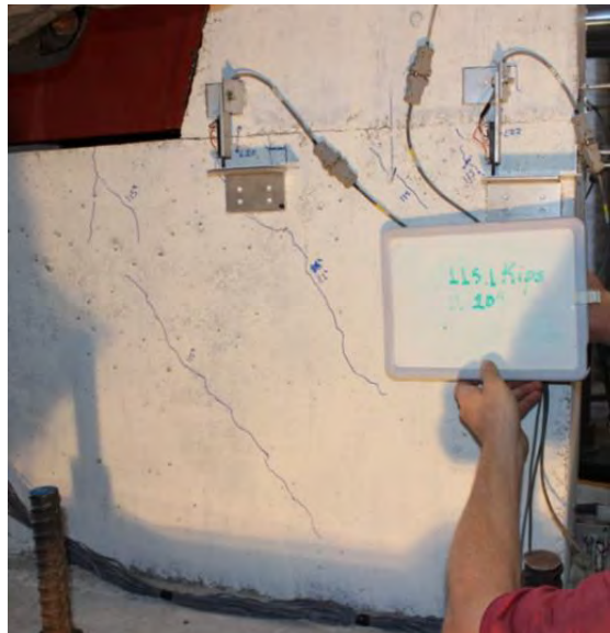
Figure 5.37 Diagonal cracks on the east side at 115-kip load in shear key 7B
