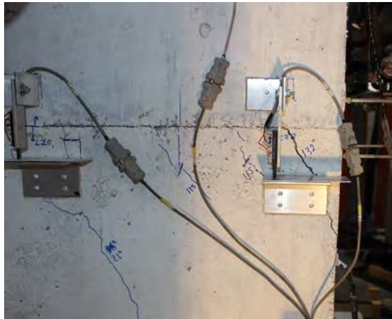
Figure 5.38 Triangular-shaped concrete piece broke off from stem wall
