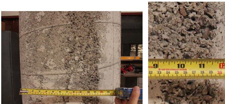
Figure 3.15 – Exposed aggregate in Pile Specimen #8
