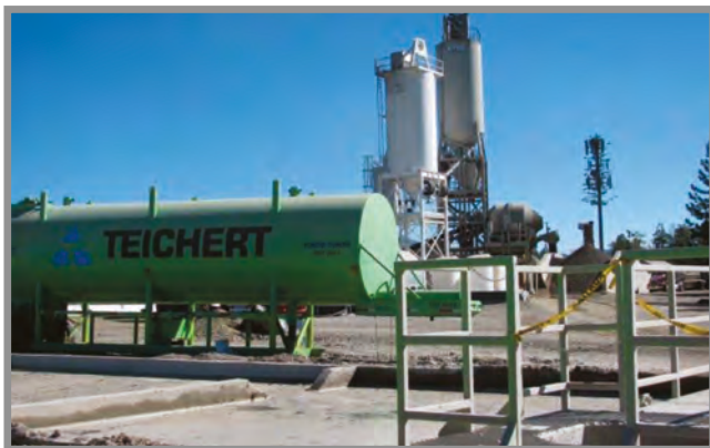
Concrete batch plant
