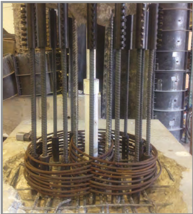
Column R-Calt-1 with couplers and new replacement longitudinal bar segments in place
