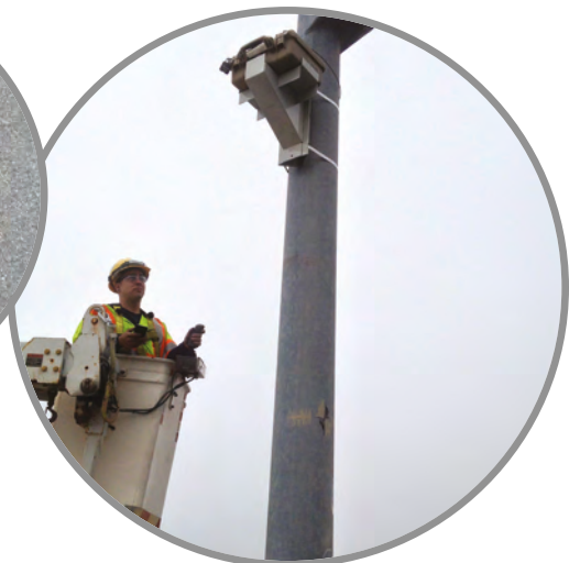
Mounting a Bluetooth detector on the crosswalk flashing beacon standard
