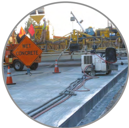
Rigid pavement reconstruction using a ternary mixture on I-80 in Emigrant Gap
