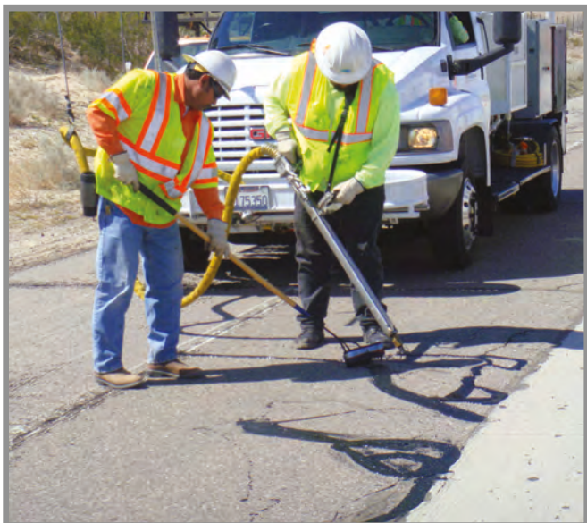
Sealzall also improves the safety of in-lane manual sealing operations because crew members are more clearly in view of oncoming traffic.
