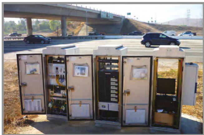
V2DVS equipment cabinets: Detection equipment (left); field PCs, one for each lane (center); server (right)
