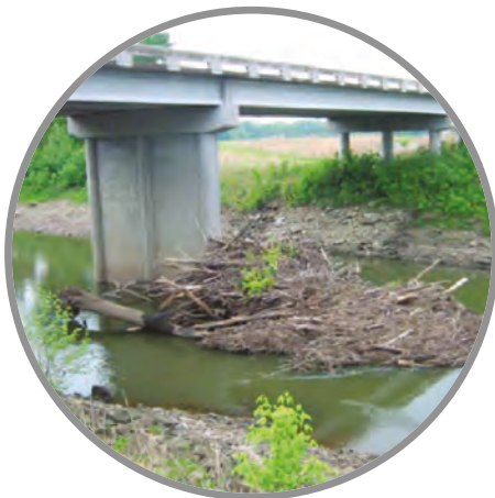
Drift accumulation on a single bridge pier (photo courtesy of Ayres Associates)
