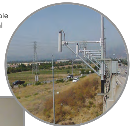
Video cameras and loops at the Sand Canyon overcrossing at the I-405 detector testbed
