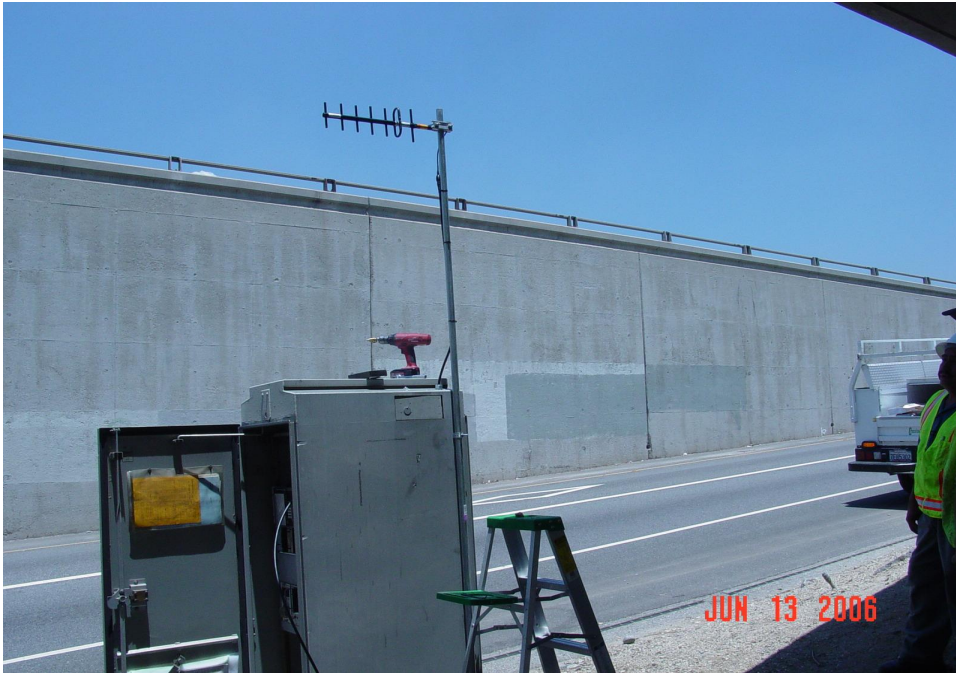
Madre St On-ramp Cabinet and Antenna
