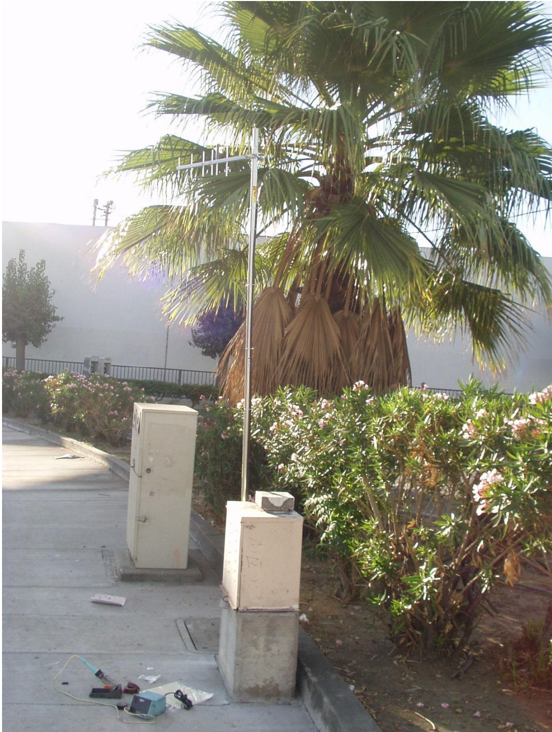
Baldwin Ave Demarcation Box and Antenna
