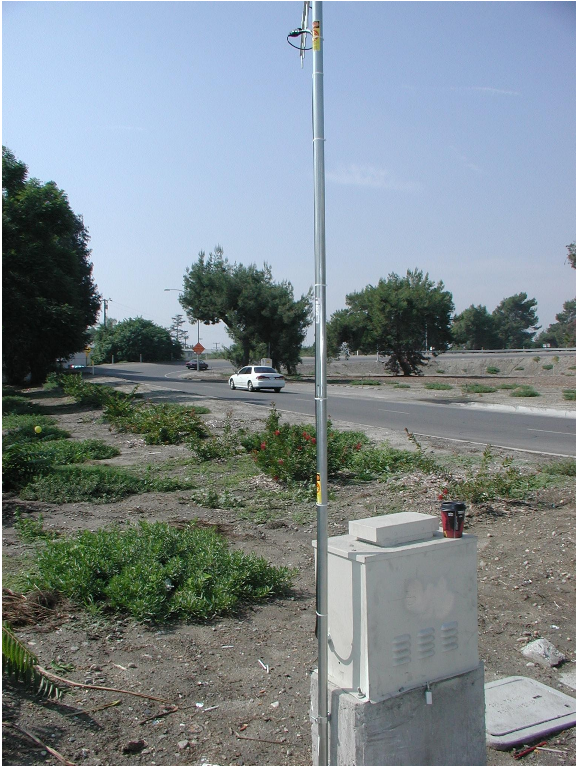
Valley Blvd Demarcation Box and Antenna
