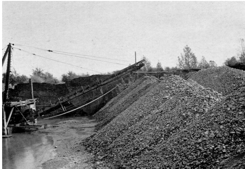
Figure 28: Dredge Tailings, Lava Beds Dredging, Butte County, 1901. Note height of tailings pile (used with permission, California Department of Conservation, California Geological Survey).
