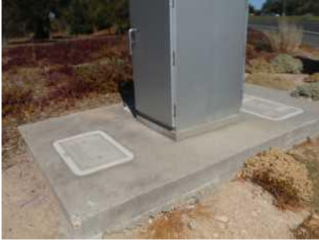
Good housekeeping at new metering station
