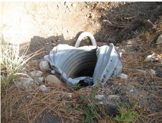
Culvert damaged scheduled for repair
