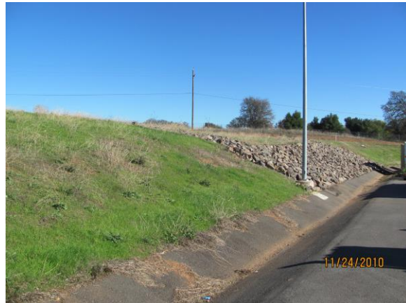
Minor slipout repaired with rock
