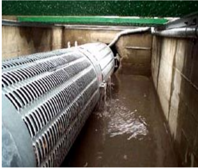
Figure C.23.6-1 Gross Solid Removal Device
