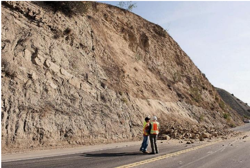
Figure C.26-1 Slopes Prone to Erosion and Sediment Discharge
