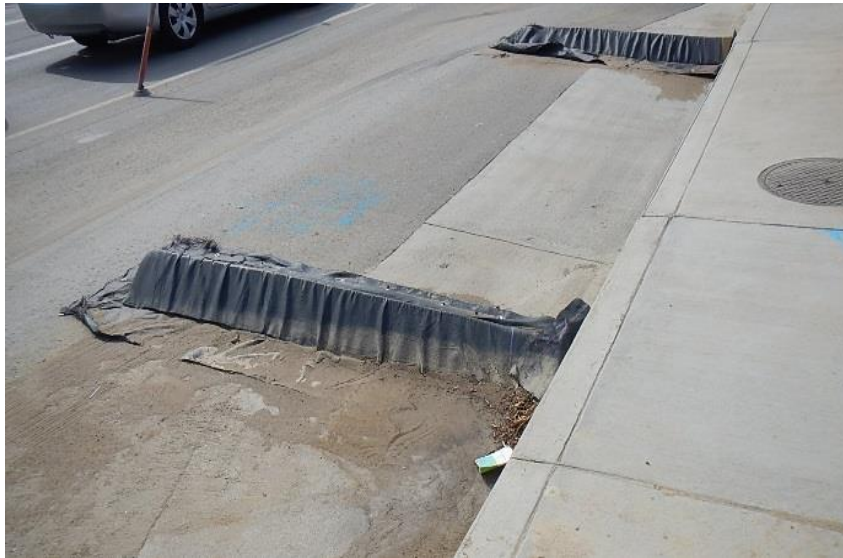
Figure C.4.9-1 Flexible Sediment Barrier
