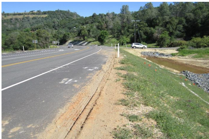
Shoulder needs stabilization after heavy winter rains
