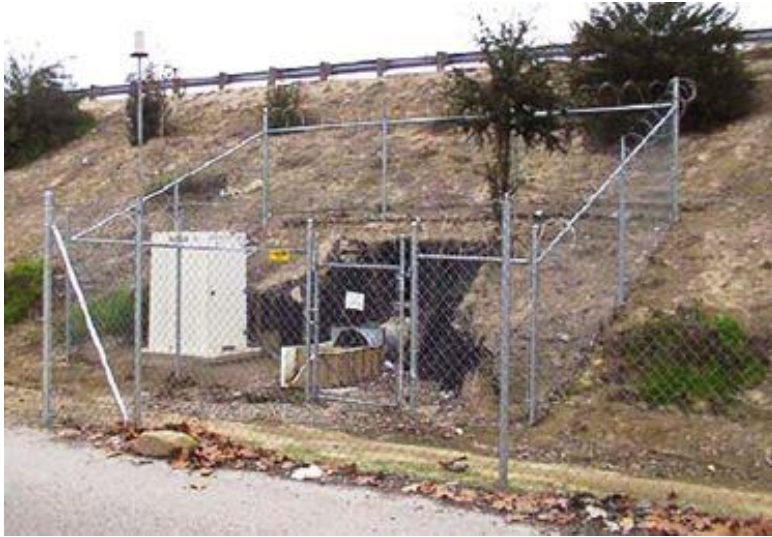
Figure 8-12 Monitoring Station Enclosed in a Secure Fence
