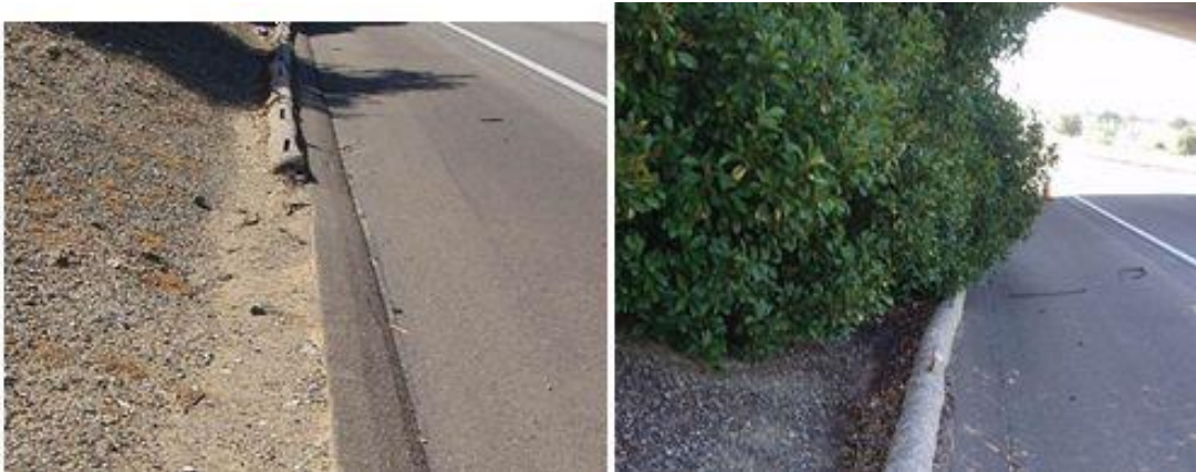
Figure 6-4 (Left) Sediment Overtopping a Curb; (Right) Overhanging Shrubbbery
