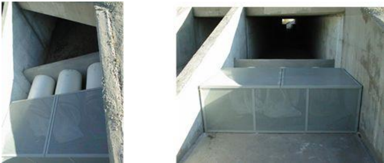
Figure 15-3 Gross Solids Monitoring Setup in Open Channels
