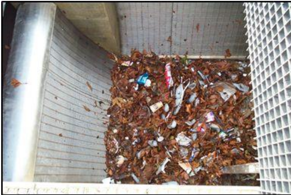
Figure 15-5 Example of Inclined Screen GSRD, View #2
