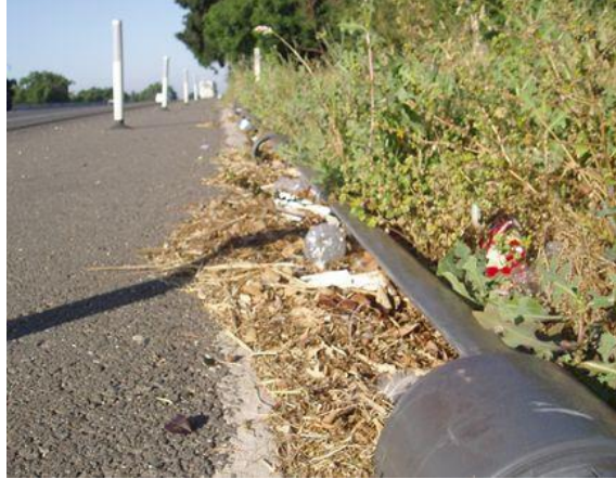
Figure 10-6 Accumulated Debris in a Stormwater Collection System
