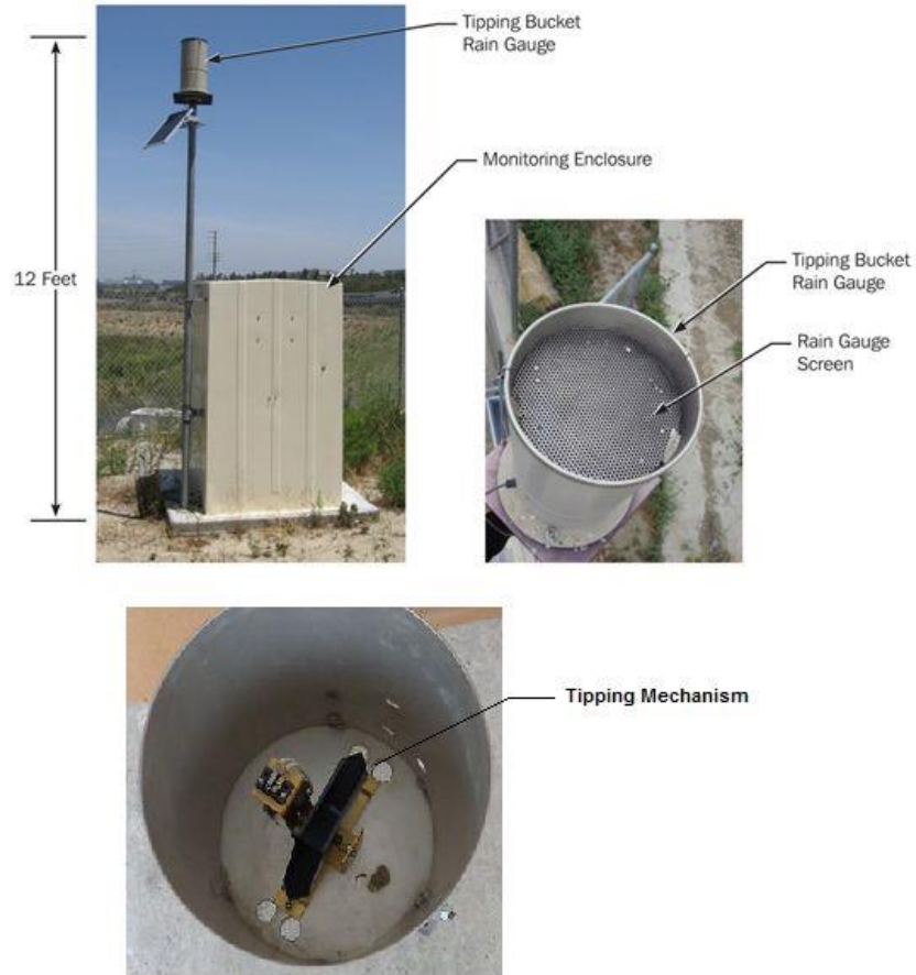
Figure 8-8 Rain Gauge Installation and Inset View
