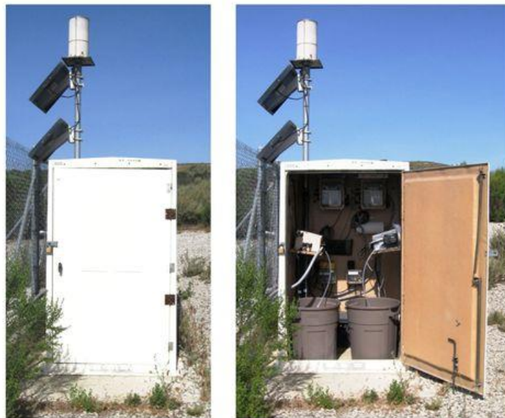
Figure 8-13 Walk-in Protective Equipment Enclosure
