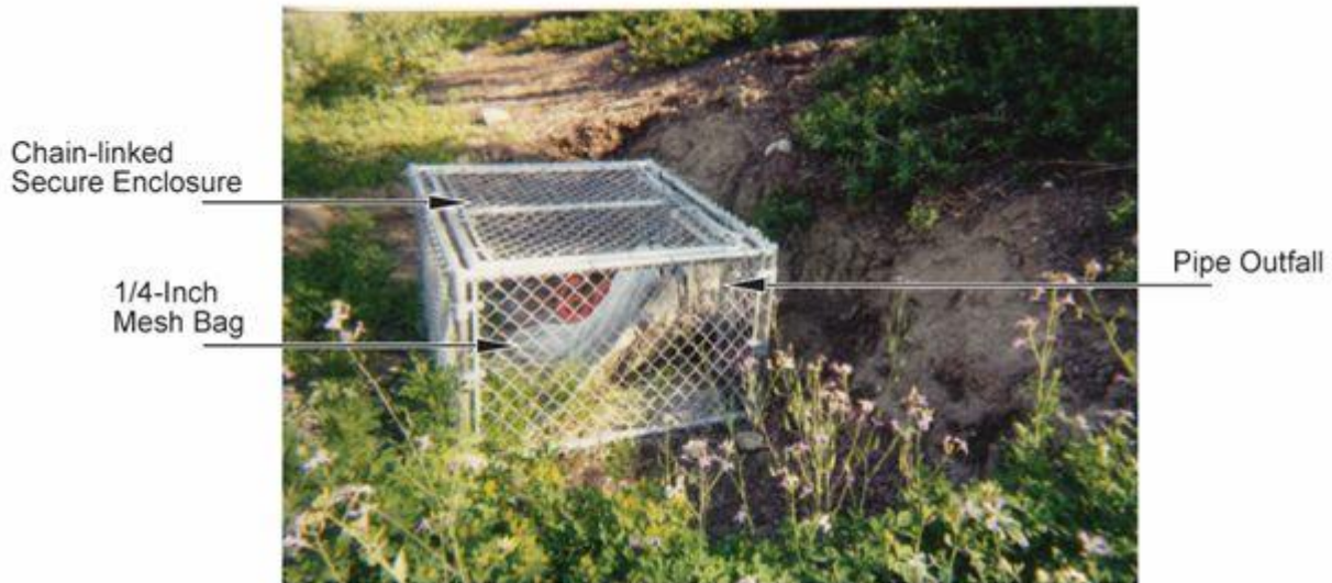
Figure 15-9 Gross Solids Monitoring Net Attached to a Pipe Outfall
