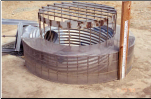
Figure 3-1 District 11 Outlet Riser
