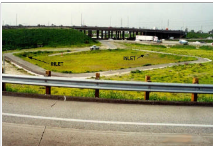
Figure 5-2 I-605/SR-91 Infiltration Basin
