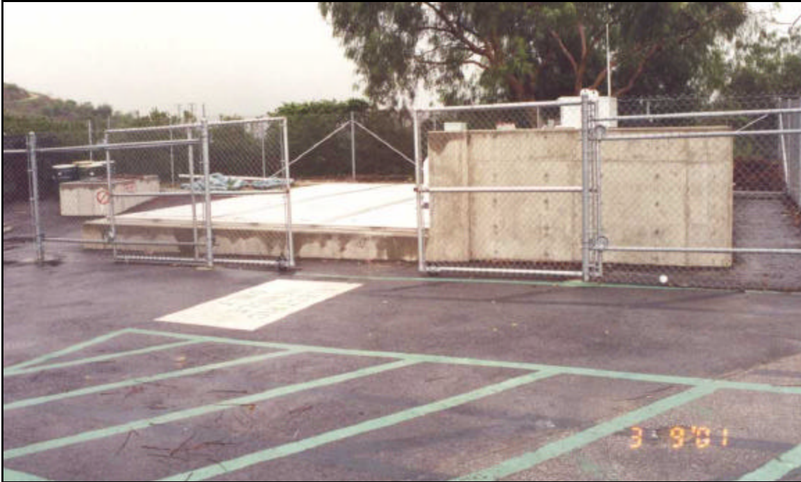
Figure 10-2 Surface View of an MCTT (Via Verde P&R)
