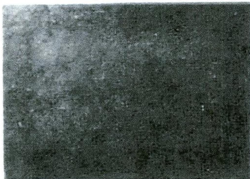
EXCESSIVE FOG SEAL OVER DGAC 0.15
