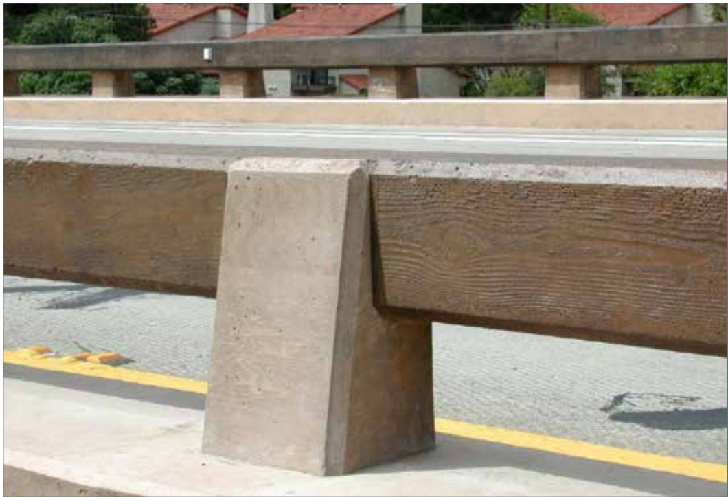
Photo of Concrete Barrier Type 80 with architectural color treatment. Sheffield Drive Bridge Demonstration Project, Santa Barbara County. (05-SB-101-PM 009.0)
