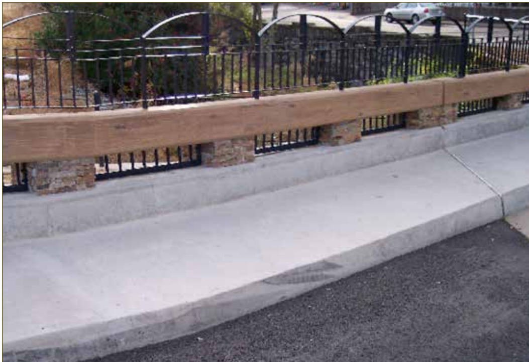
Interior view of Concrete Barrier Type 80SW with architectural treatment and modified pedestrian railing at the Canal Street Bridge at the Highway 49/50 Junction in Placerville, El Dorado County. (03-ED-050-PM 017.52)
