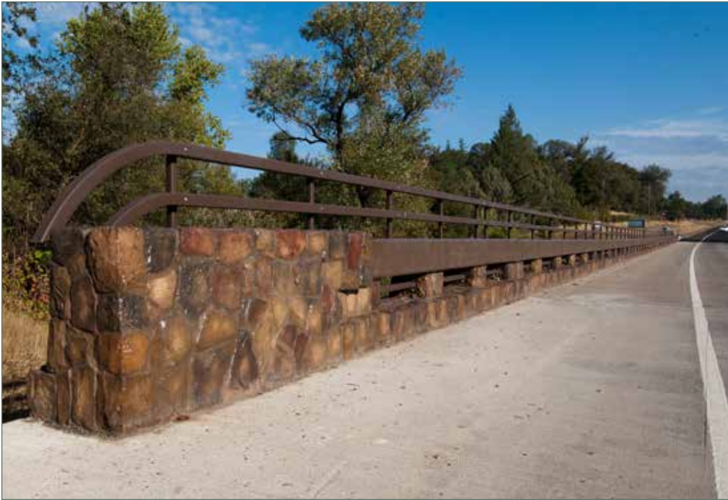
View from bridge approach slab of Concrete Barrier Type 80 with architectural treatment and 54-inch-high bicycle rail offset 15 inches from barrier rail face on the Bear River Bridge on the Placer/Nevada County line. (03-PLA-049-PM 011.35)
