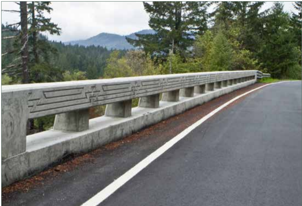
Photo of Concrete Barrier Type 80 on barrier moment slab over retaining wall with tribal design architectural texture in Humboldt County. (01-HUM-096)
