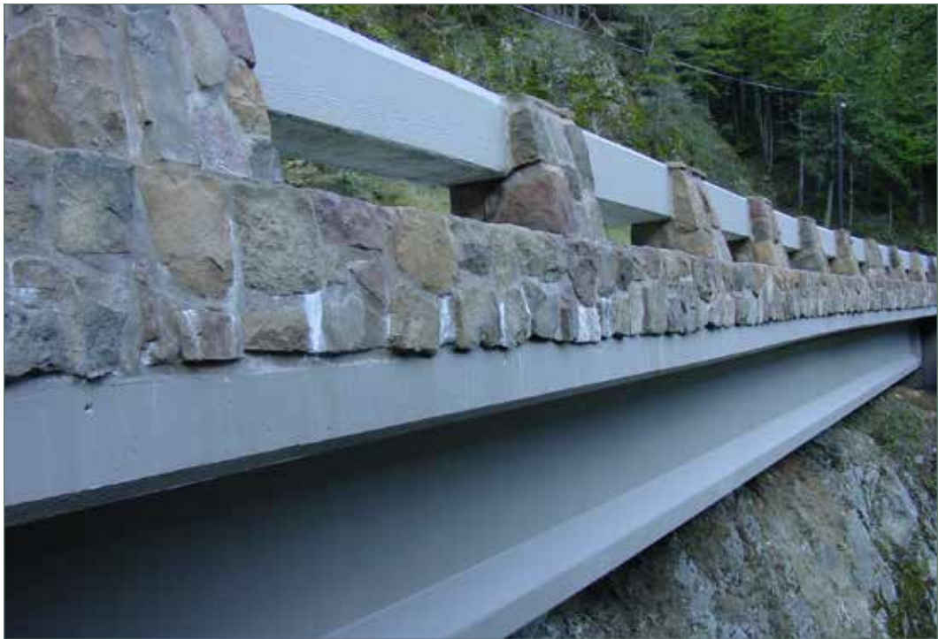
Photo of exterior view of Concrete Barrier Type 80 modified with architectural treatment at Myrtle Creek Sidehill Viaduct in Del Norte County. (01-DN-199-PM 007.32)
