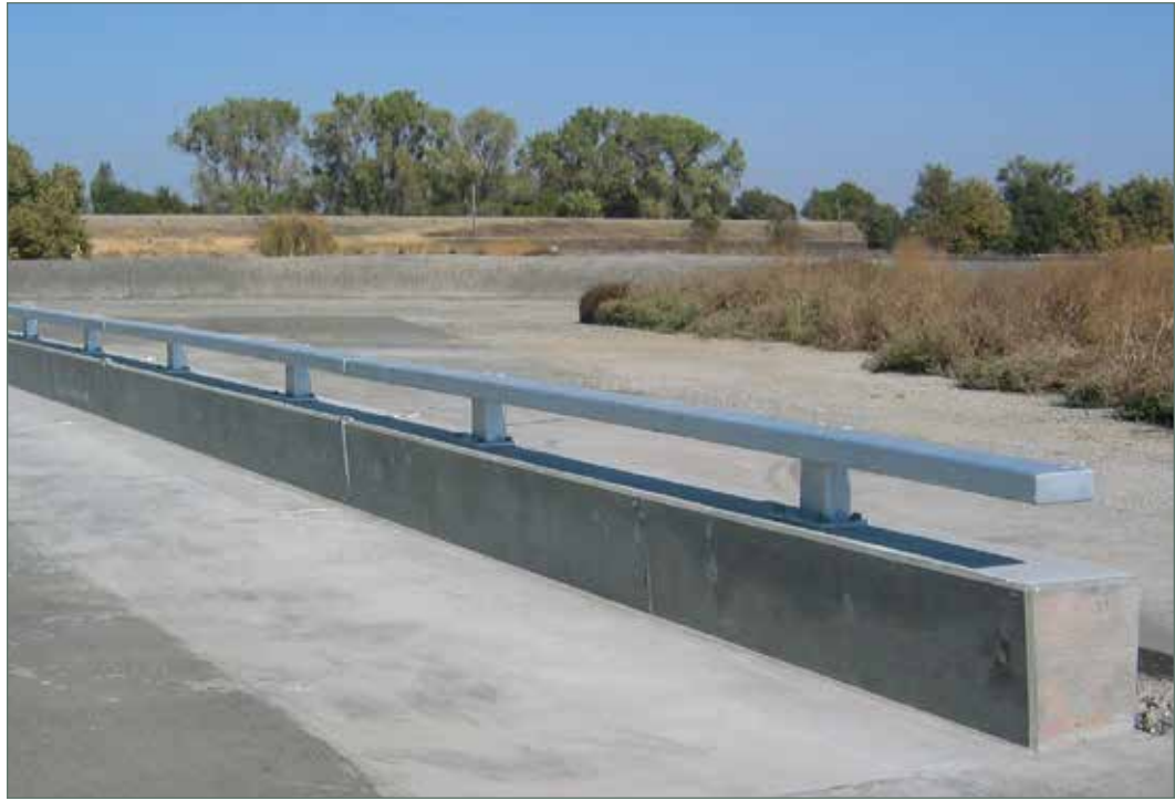
Concrete Barrier Type 90. As of June 2011, this new bridge barrier type had not been used on a bridge. Photos are from the crash test site; consequently, there are no full-height concrete anchor blocks at the ends of the barrier.
