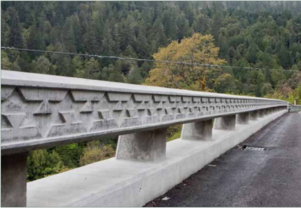
Concrete Barrier Type 80 on barrier moment slab over retaining wall with tribal design architectural texture in Humboldt County. (01-HUM-096)
