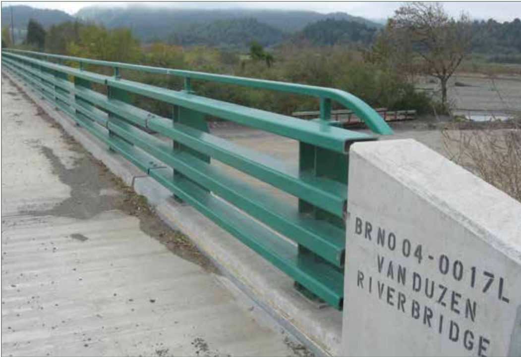
Photo of California ST-20S Bridge Rail painted green at Van Duzen River Bridge in Humboldt County. (01-HUM-101-PM 056.8)
