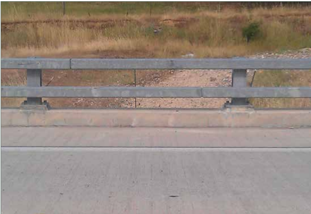
Photo of interior view of California ST-30 Bridge Rail at the South Fork Dibble Creek Bridge in Tehama County. (02-TEH-036-PM 39.0)
