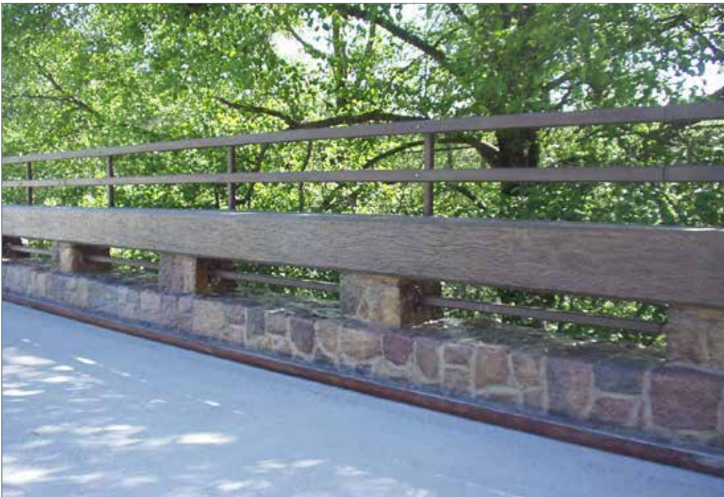
Photo of Concrete Barrier Type 80 with architectural treatment and bicycle rail offset 15 inches from rail face on the Bear River Bridge at the Placer/Nevada County line. (03-PLA-049-PM 011.35)
