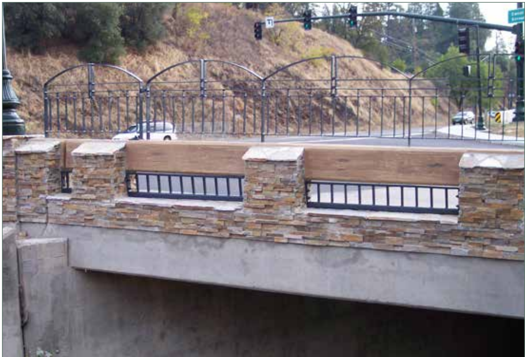
Exterior view of Concrete Barrier Type 80 with architectural treatment and modified bicycle railing at Canal Street Bridge at Highway 49/50 junction in Placerville, El Dorado County. (03-ED-050-PM 017.52)
