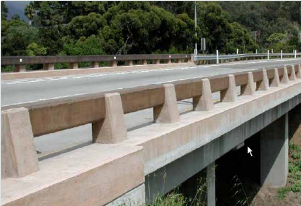
Photo of Concrete Barrier Type 80 modified with color treatment. Sheffield Drive Bridge, Santa Barbara County. (05-SB-101-PM 009.0)
