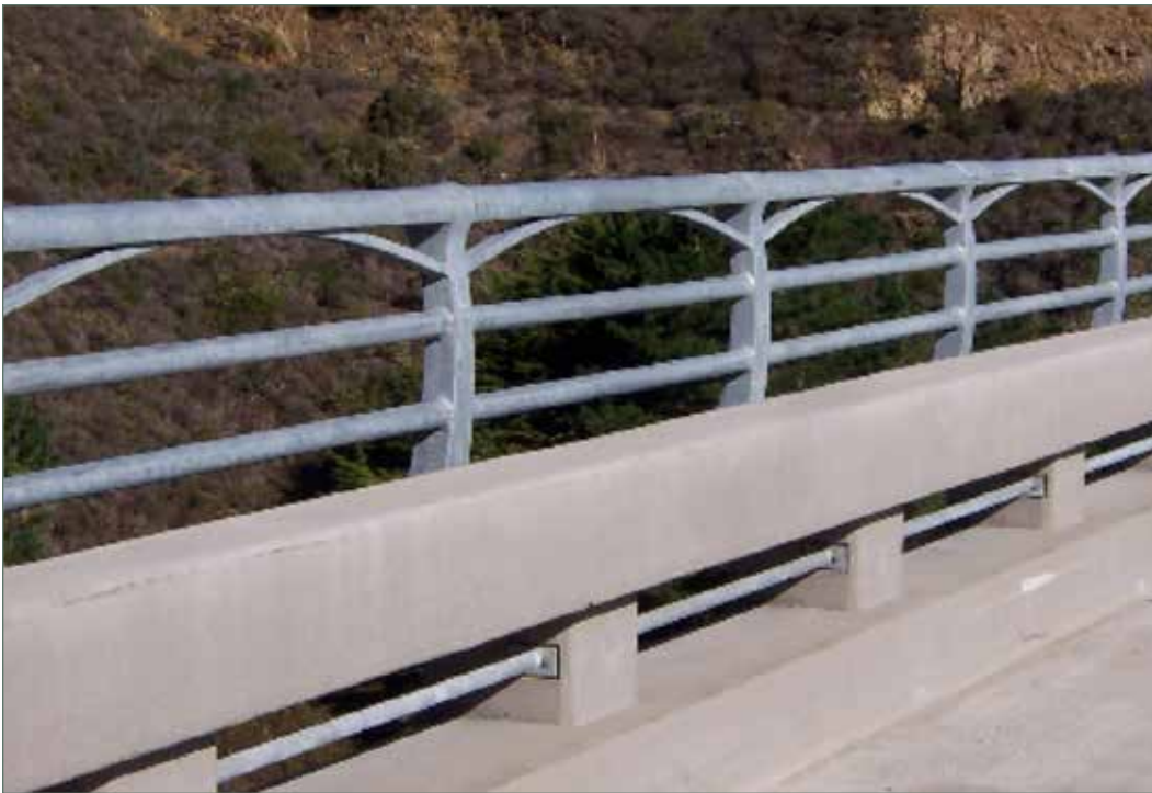
Photo of Concrete Barrier Type 80 with 54-inch-high bicycle rail offset 15" from rail face on the completed Devil's Slide Bridge at North end of Devil's Slide Tunnel in San Mateo County. (04-SM-001-PM 39.66)
