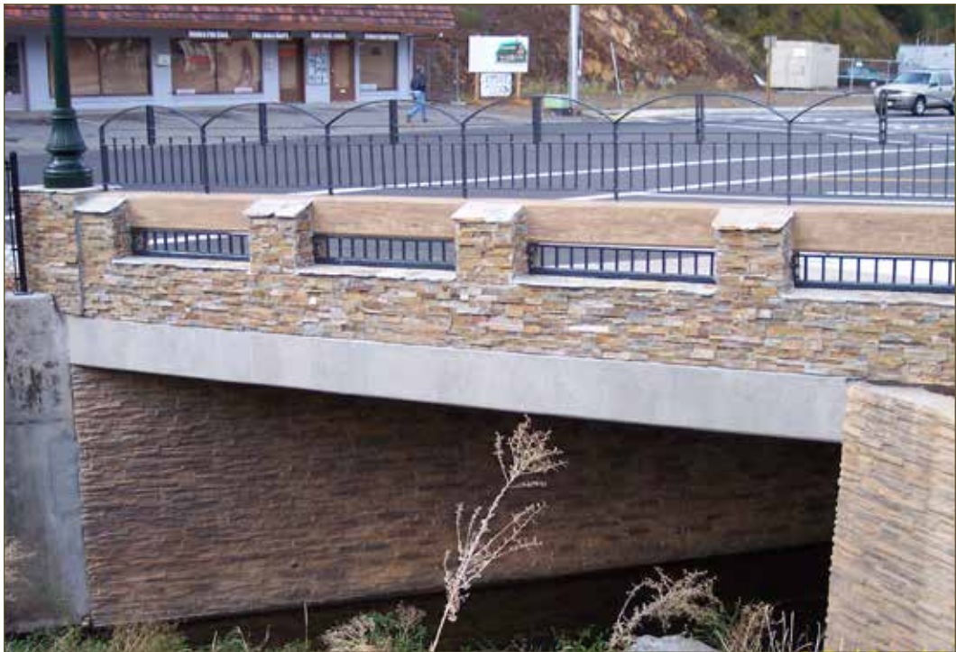
Exterior view of Concrete Barrier Type 80SW with architectural treatment and modified pedestrian railing at the Canal Street Bridge at the Highway 49/50 Junction in Placerville, El Dorado County. (03-ED-050-PM 017.52)
