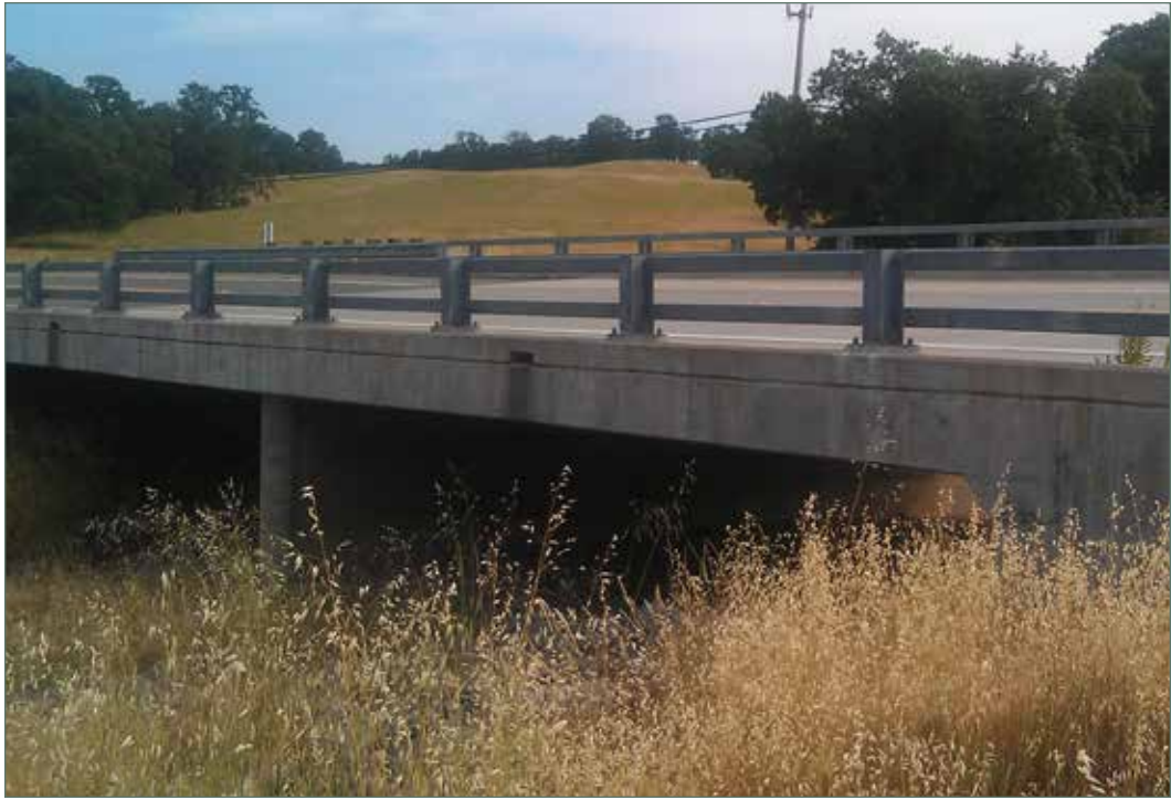
Photo of exterior view of California ST-30 Bridge Rail at the South Fork Dibble Creek Bridge in Tehama County. (02-TEH-036-PM 39.0)
