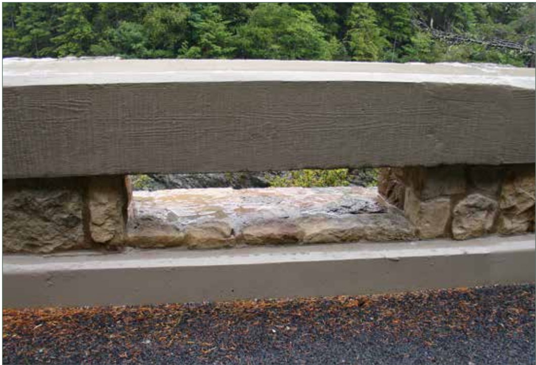
View from sidehill viaduct bridge deck of Concrete Barrier Type 80 with architectural texture and color at the Myrtle Creek SideHill Viaduct in Del Norte County. (01-DN-199-PM 007.32)
