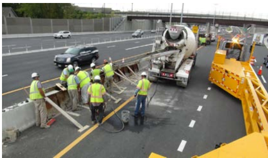
Concrete Barrier Construction Using Mobile Barrier System for Positive Protection Photo Source: Mobile Barriers LLC
