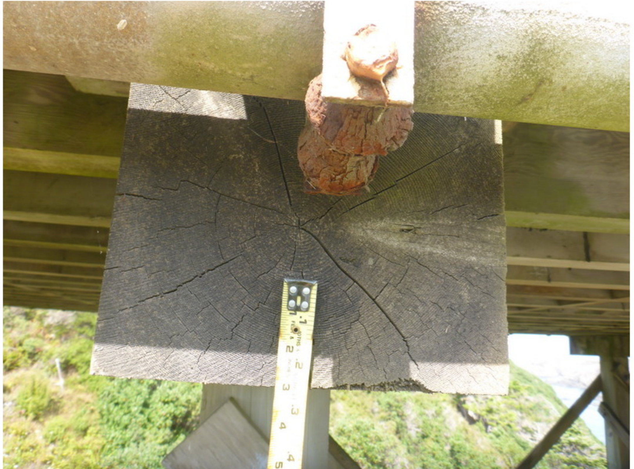
Photo No. 16 Typical checks visible at the end of the bent caps.
