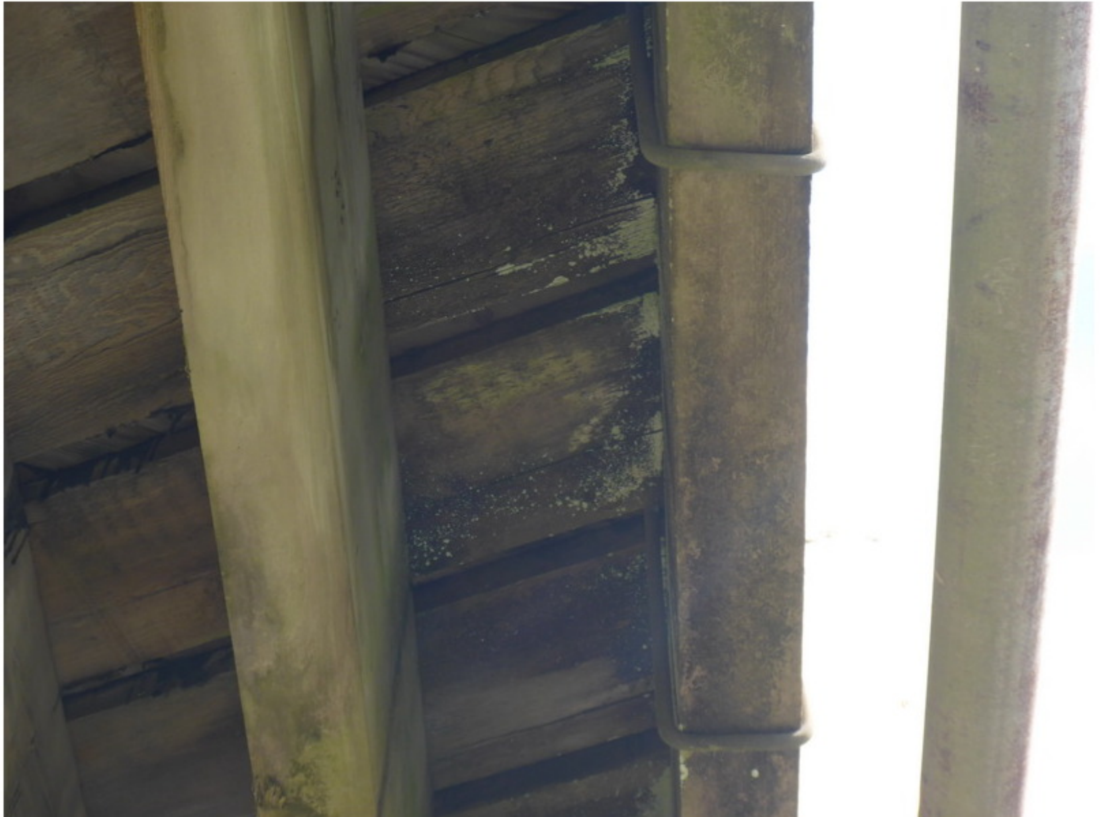
Photo No. 1 Typical mold and rot located along the edges of the timber deck.
