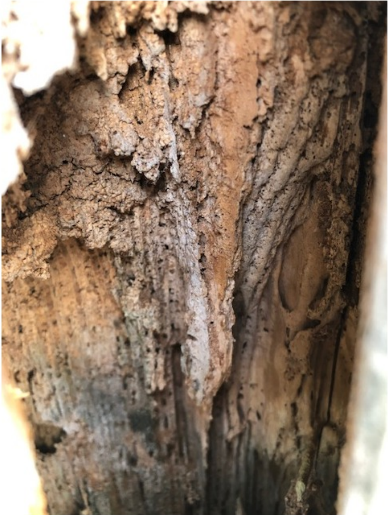
Photo No. 13 Core rot due to termites in Column 4 at Bent 23.
