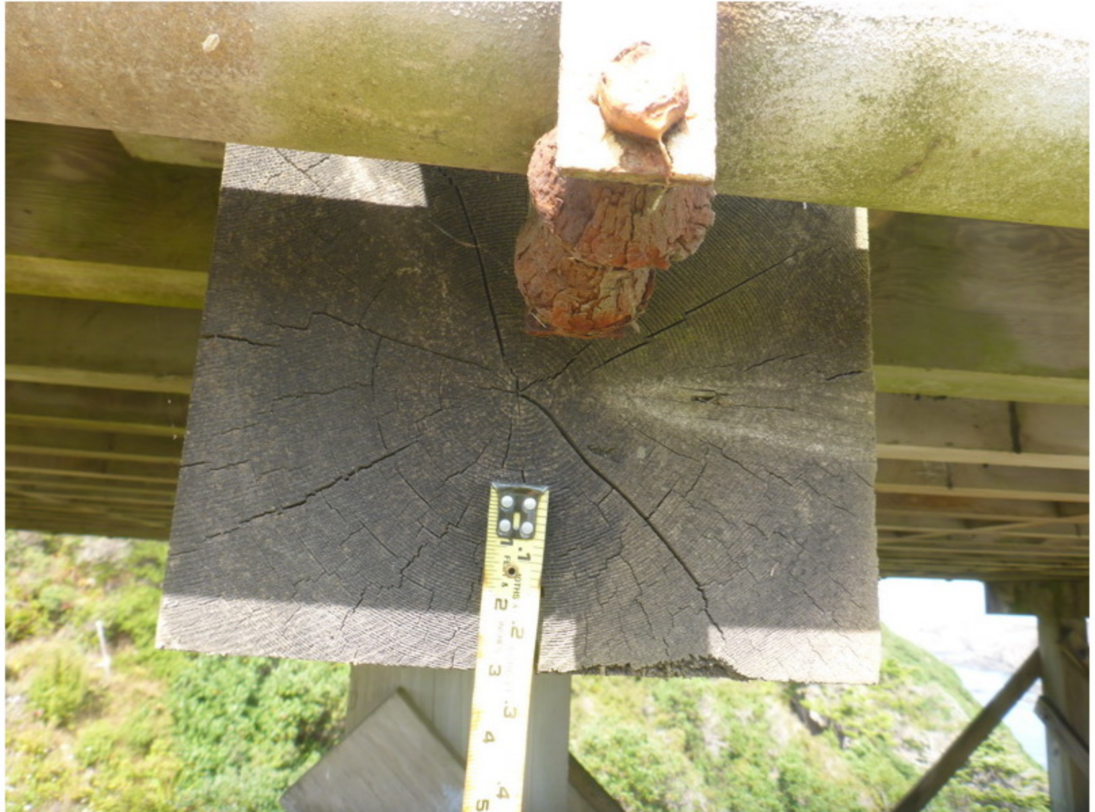
Photo No. 16 Typical checks visible at the end of the bent caps.
