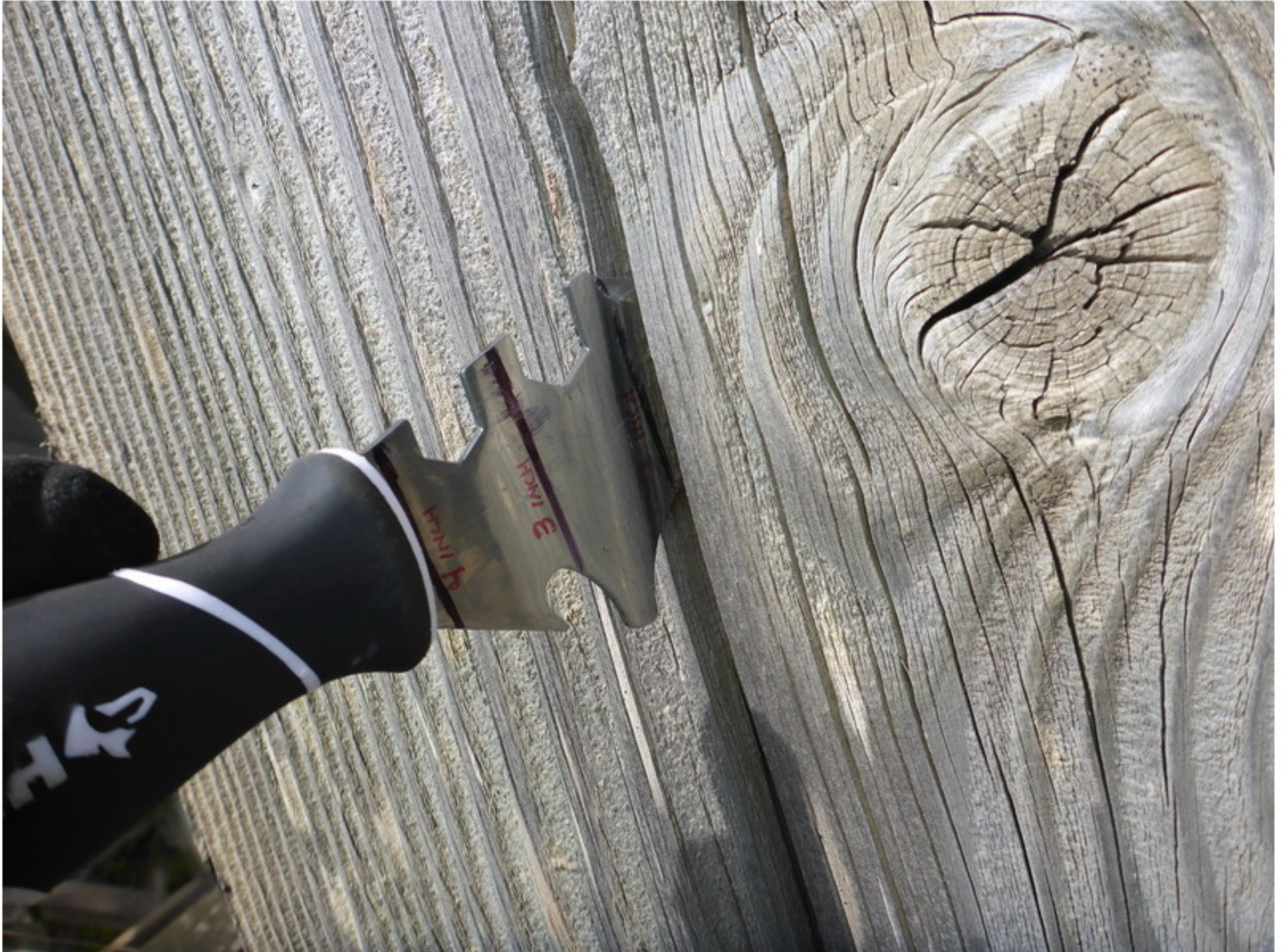
Photo No. 11 Large check along the fourth column of Bent 9.
