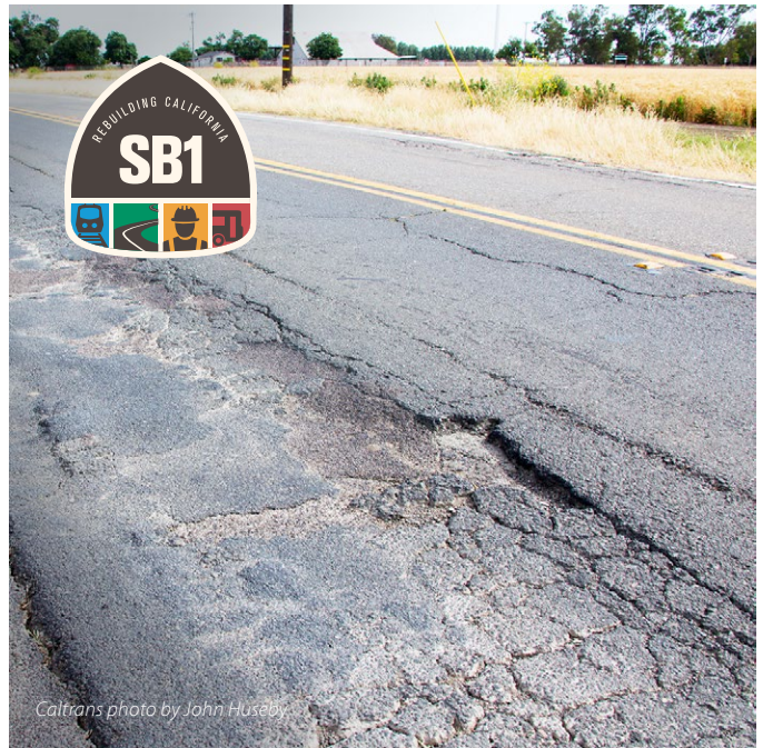
Roads in need of repair such as Highway 113 in Yolo County will be fixed sooner after the CTC agreed to expedite pavement repair projects.
