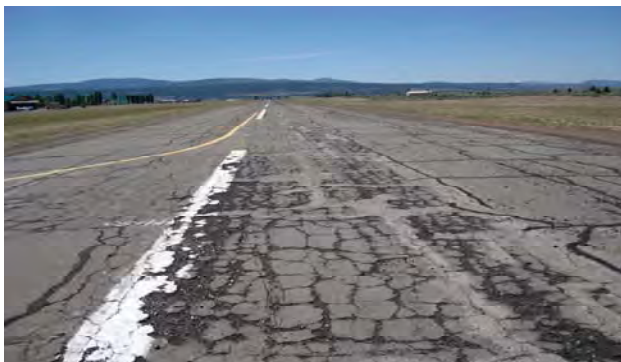
Before: Failed Pavement (Rwy 5)
