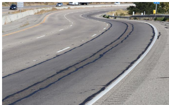
Section of U.S. Highway 101 north of Gaviota in Santa Barbara County before striping project.
