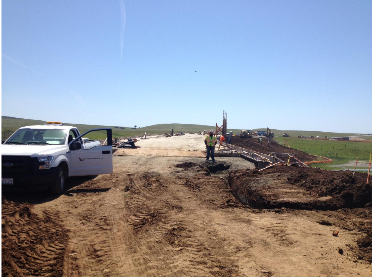
Bridge Deck and Earthwork at Arroyo Del Corral Creek as part of State Route 1 Realignment Project.
