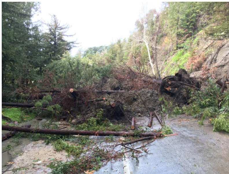
Slide activity on State Route 1 in Monterey County resulting in downed trees, mud and rocks.
