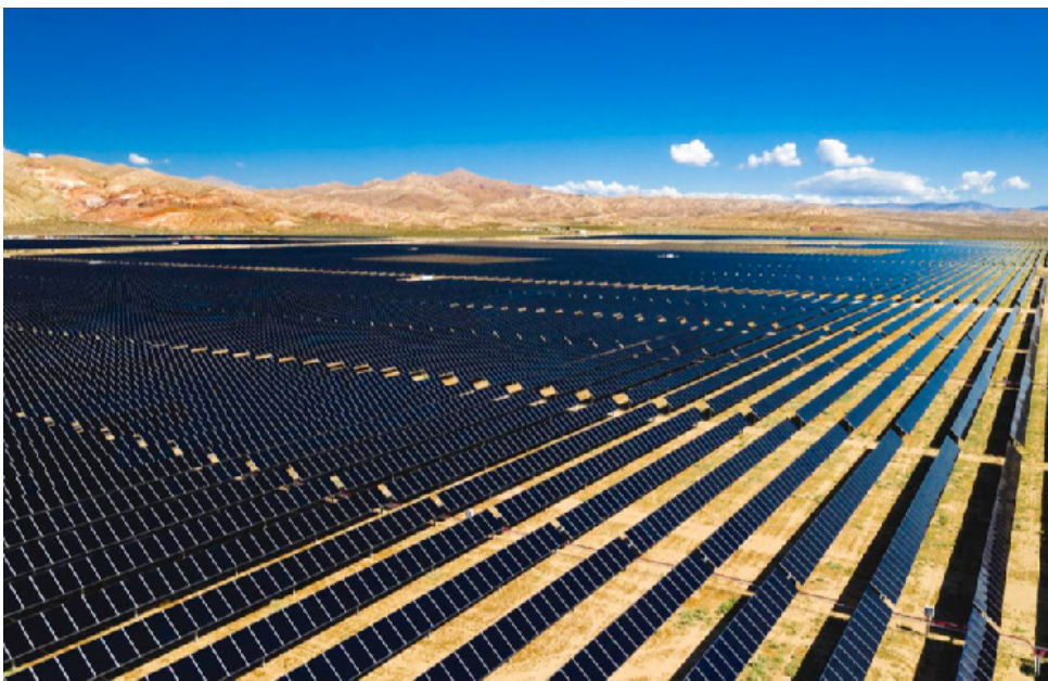
8minute Solar Energy’s 121-megawatt Solar Farm was completed in 2019 in Cantil. It was the first phase of a 1,500-acre project that began in 2015. The farm provides electricity to power more than 150,000 homes in the Los Angeles metro area.
