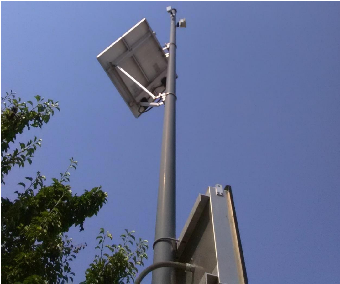
Figure 18 - Sensys repeater mounted on Trailblazer sign pole
