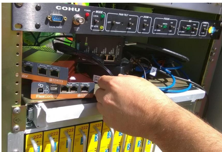
Figure 24 - Sensys equipment in ramp meter cabinet
