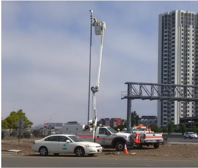
Figure 15 - mounting a Sensys repeater on the CCTV pole
