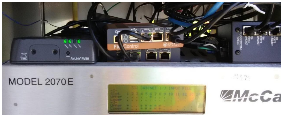
Figure 25 - Sensys equipment in traffic signal cabinet
