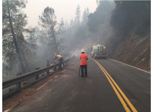
The Helena Fire in August and September 2017 burned the area around SR 299 in Trinity County. (credit: Caltrans District 2)
