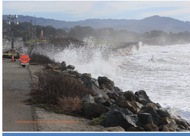
ROADWAY EXPOSURE TO TIDAL FLOODING, SURGE, AND EROSION
