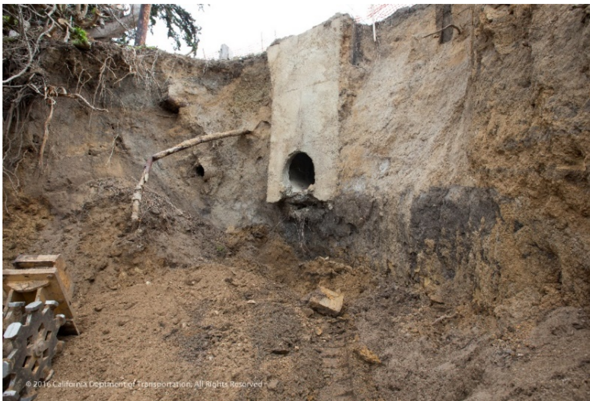
DAMAGED CULVERT UNDER REPAIR IN DISTRICT 4
