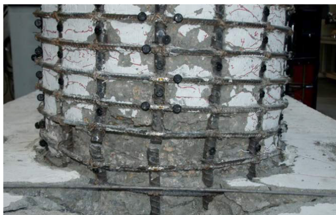
FIGURE 5: final damage state
