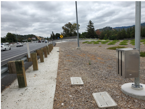
Image 4: TIRTL transmitter and adjacent CCTV camera pole at the South Main Street count station location
