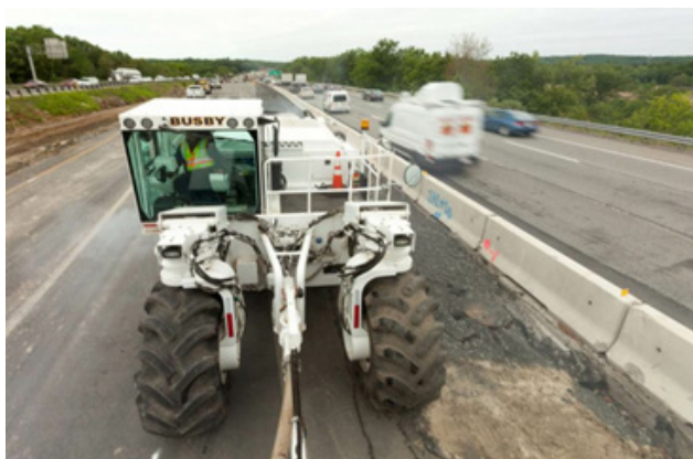
Image 1: Full depth reclamation offers a number of benefits, including minimal traffic disturbance, environmental friendliness and minimal use of virgin material. Photo courtesy of Roadtec
