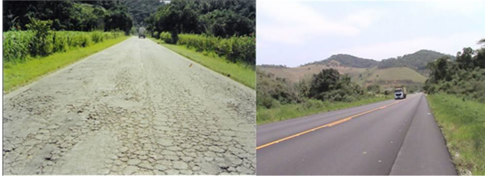
Figure 2.12: Highway RJ-122 pavement in Brazil before and after overlay placement with an ARFC surface.
