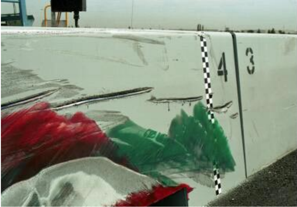
Figure 2-19 Barrier face gouges from vehicle lug nuts after Test 572
