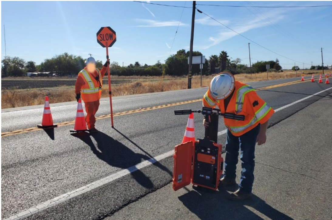
Figure 5.26 Location of AWARE Sentry Deployment at Flagger Location 1
