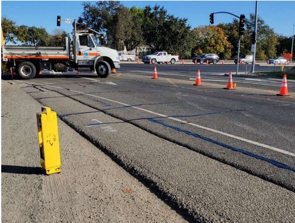
Figure 5.34 Deployment of Single Sentry Beam within Closure on On-Ramp
