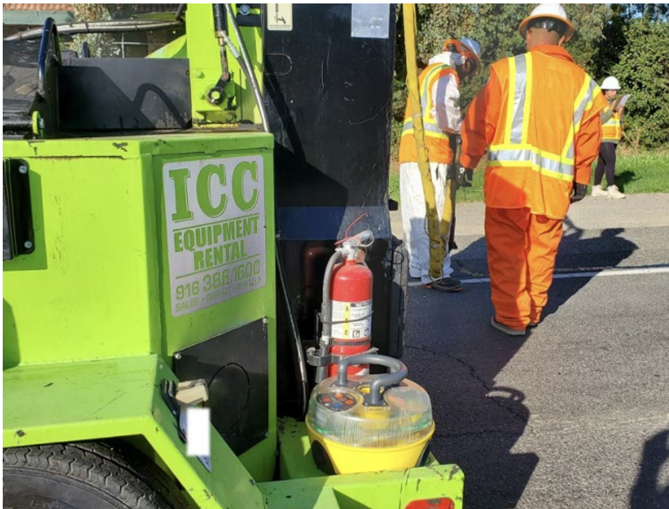
Figure 5.35 Location of Intellicone PSA Deployment on Maintenance Vehicle
