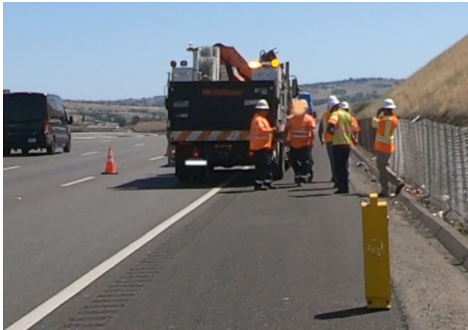
Figure 5.12 Location of Single Sentry Beam Deployment inside the Work Zone
