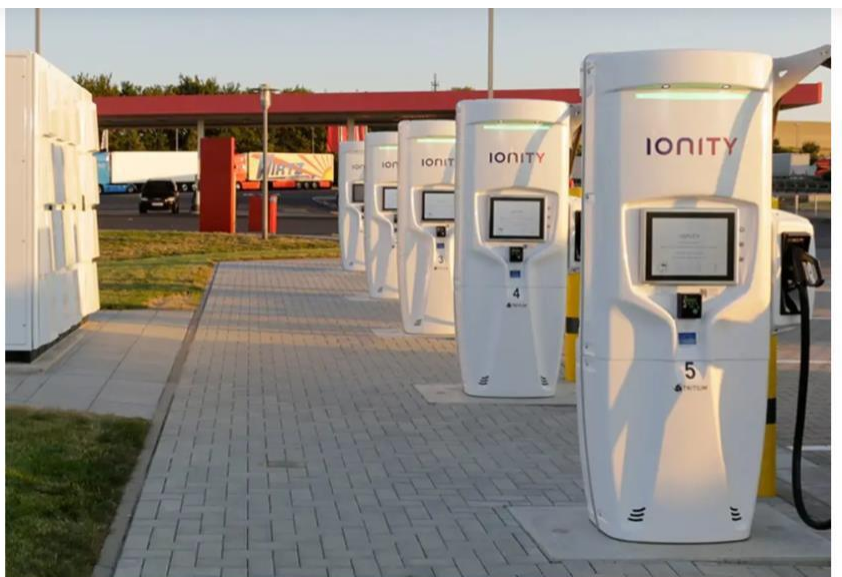
Figure 14. A rectifier with multiple chargers
