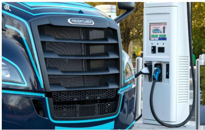
Figure 12. A truck connected to a high power charger
