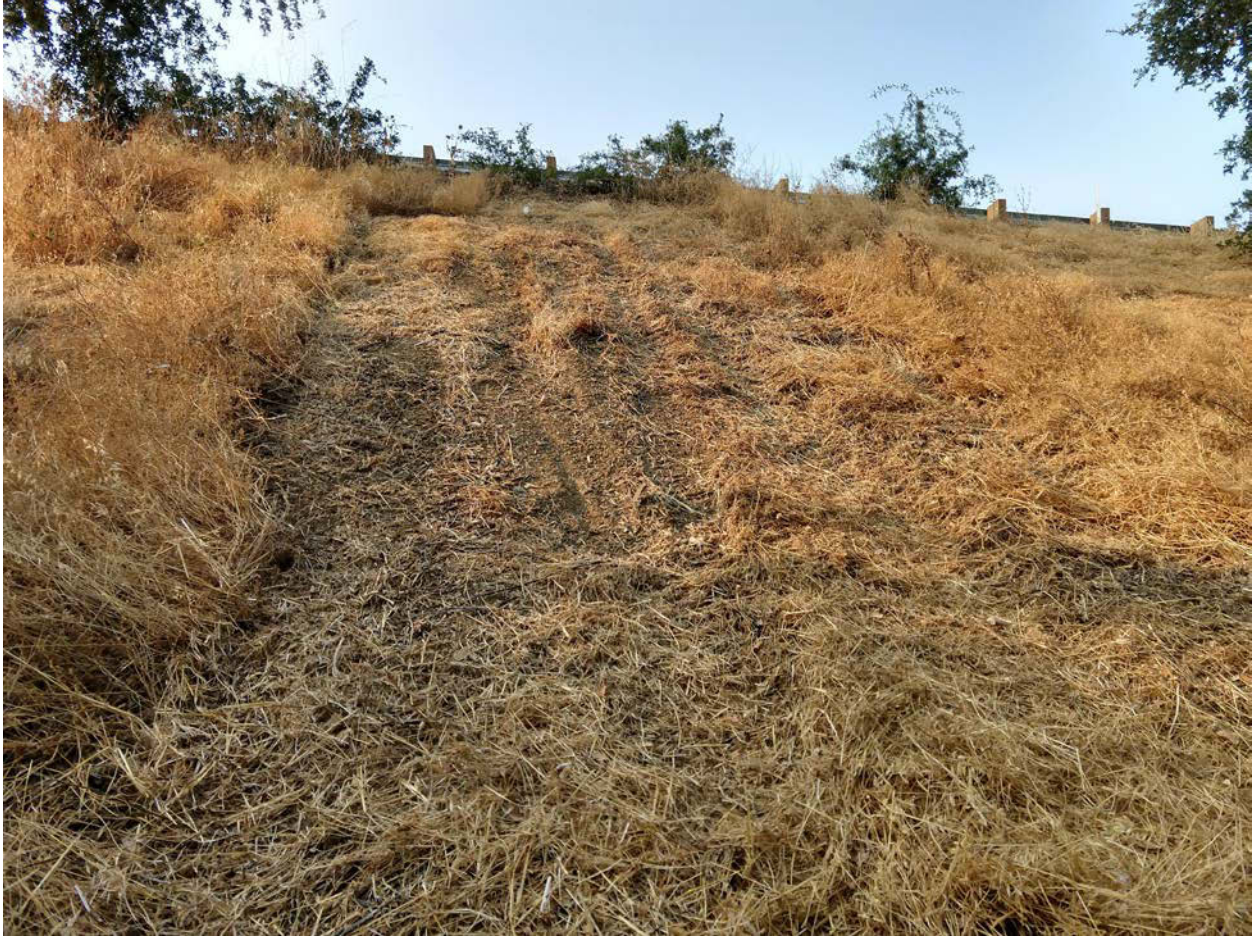
Figure 5.6: Close-up view of erosion on ground without mulch
