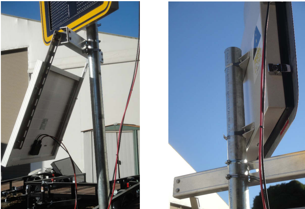
Figure 4.6 VSA sign and solar panel wire connection
