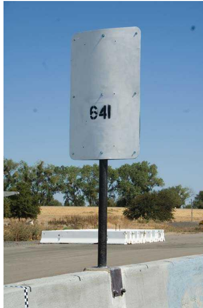
Figure 2-2 Signpost Mounted on Type 60 Median Barrier
