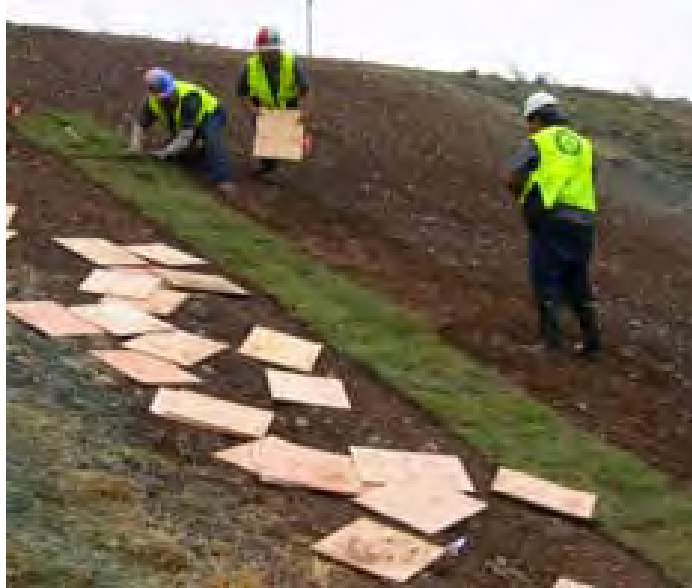
Figure 5.21 Placing MSU Native Grass Sod–Hedgerow on the highway fill-steep slope area in November 2006.
