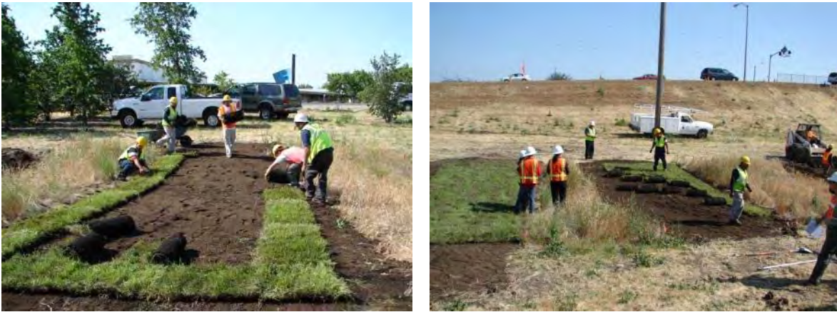
Figure 5.24 Installation of MSU Native Grass Sod–Delta on the highway drainage swale test area in May 2008.
