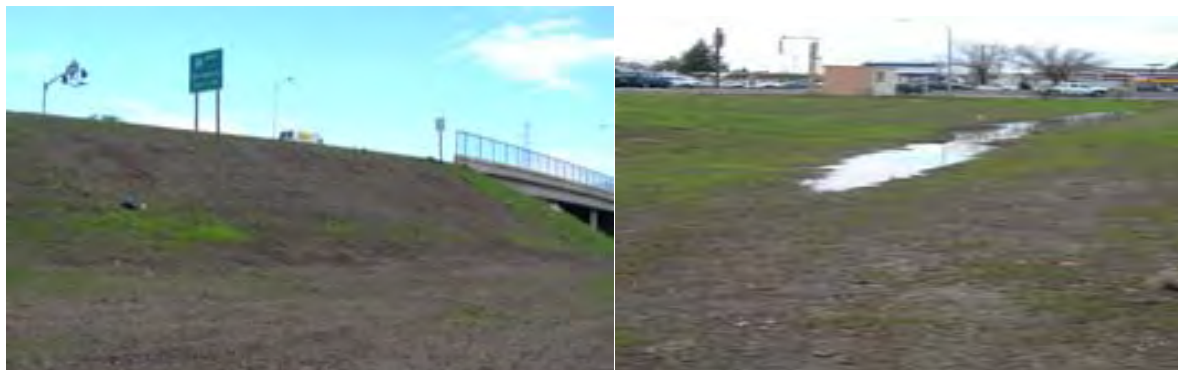
Figure 5.15 Highway fill-steep slope (left photo) and drainage swale (right photo) located at the Mack Road and Highway 99 intersection.
