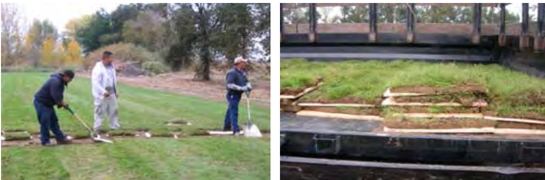
Figure 5.20 Lifting the cut sod onto boards using a shovel (left photo) and stacking the boards for transport on a trailer bed (right photo).
