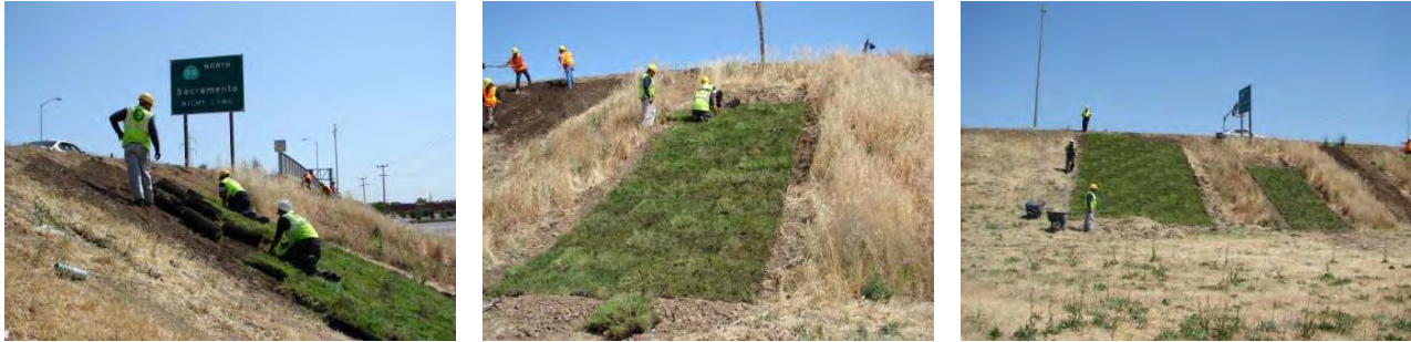
Figure 5.23 Installation of MSU Native Grass Sod–Delta on the highway fill-steep slope test area in May 2008.
