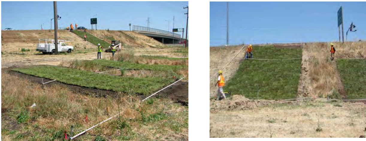
Figure 5.26 Irrigation line installation following transplanting the MSU Native Grass Sod–Delta on the drainage swale (left photo) and steep slope (right photo) areas on May 7, 2008.
