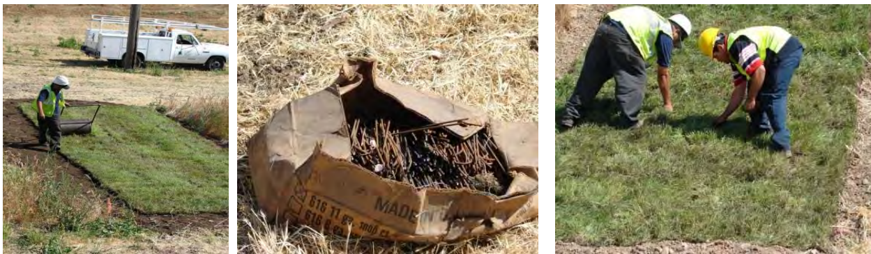
Figure 5.25 Installed sod was rolled to enhance contact with underlying soil (left photo), then staples were inserted by hand to hold sod in place (middle and right photos).
