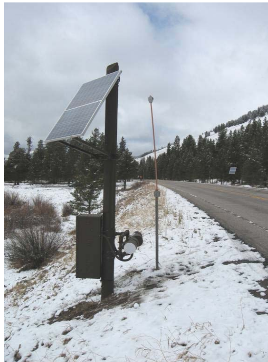
Figure 2.8: Station 11 at its new location, looking north (Detection Zone C) towards Station 15 and Black Butte Trail parking area (Photo: Marcel Huijser, WTI-MSU)
