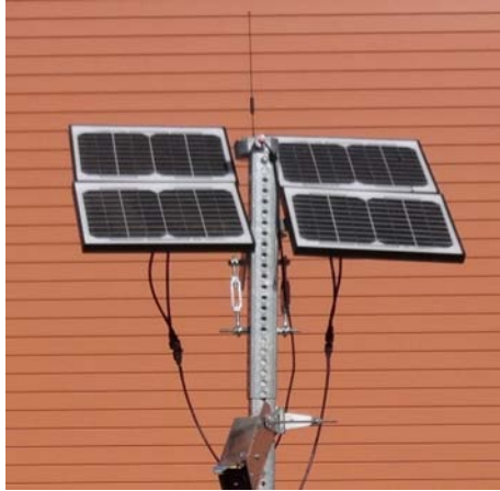
Figure 121 Mounted solar panel arrangement (ALEK0® 10W Monocrystalline solar panel).
