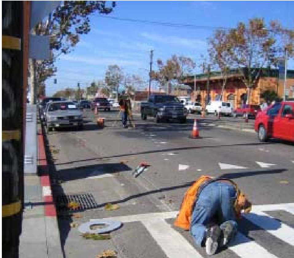
Figure 17 East 14 th Street Installation: Survey and Mark (1m around station, 10m otherwise) on the Ground
