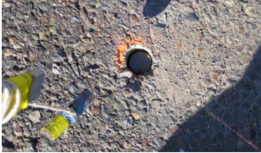
Figure 21 East 14 th Street. Installation: Placing Magnet and Checking Polarity (with home-made tool)
