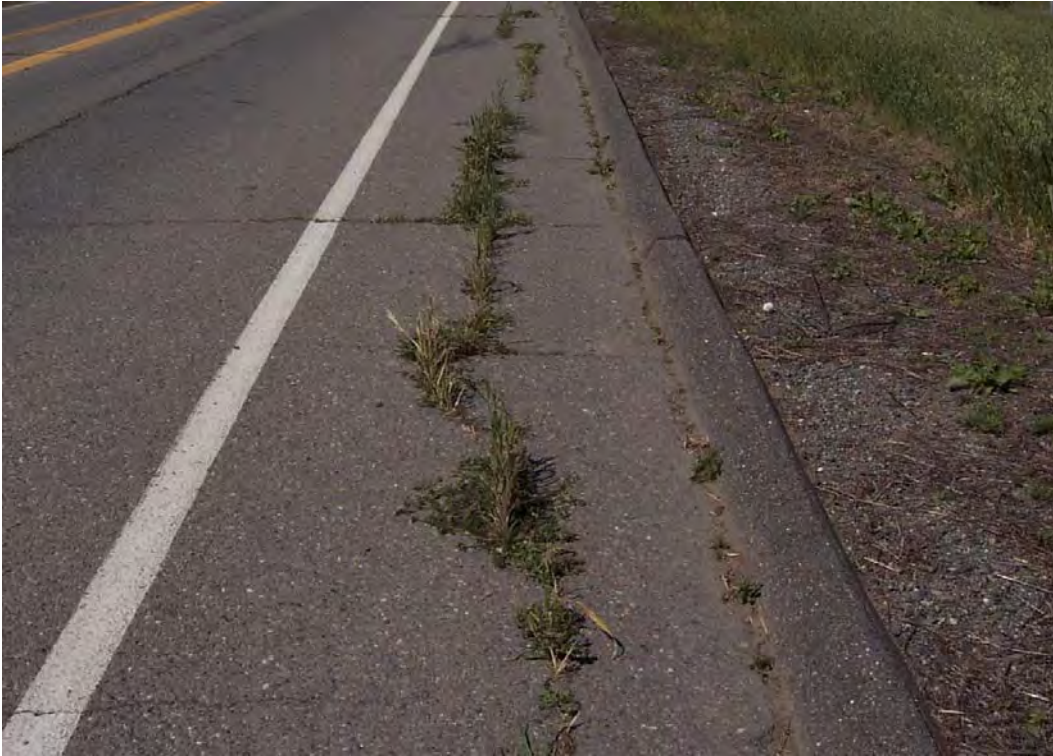
Figure 2.5 Urban Vegetation in Roadway Crack
