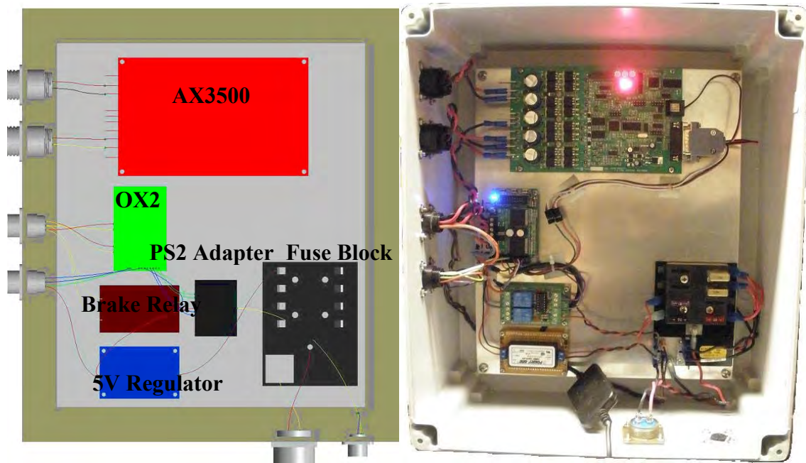
Figure 6.7: NEMA Box Pro/Engineer Model (left), Actual NEMA Box wiring (right)
