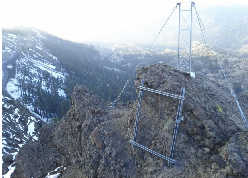
Figure 3.6: The west view of the final site tower installation and electronics enclosure mounting brackets
