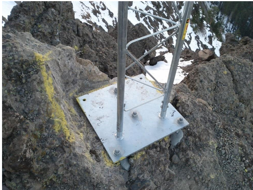
Figure C.3: The tower base bolted to the rock conglomerate
