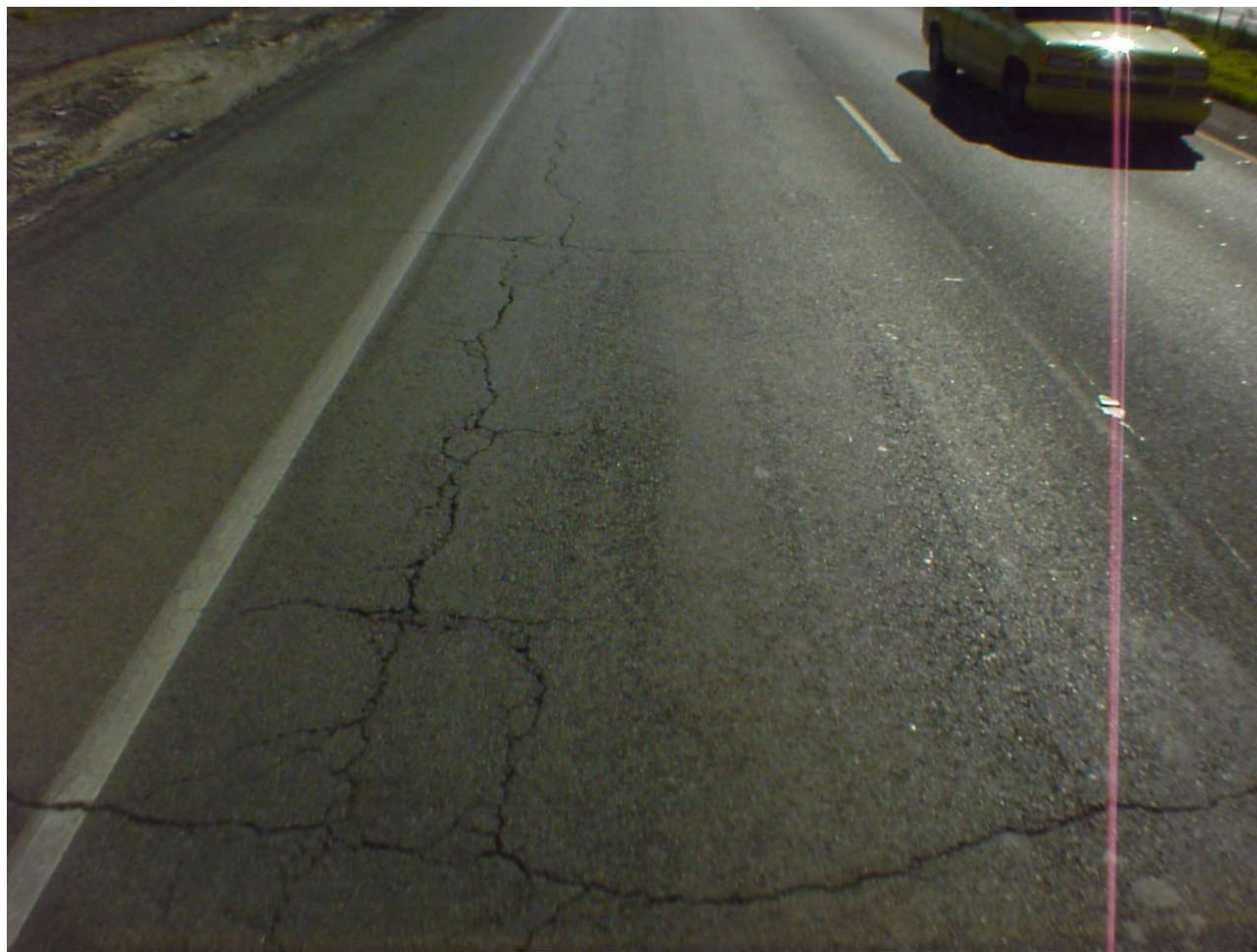
Figure 8-15: Example Distresses on SC Zone RAC Sections
