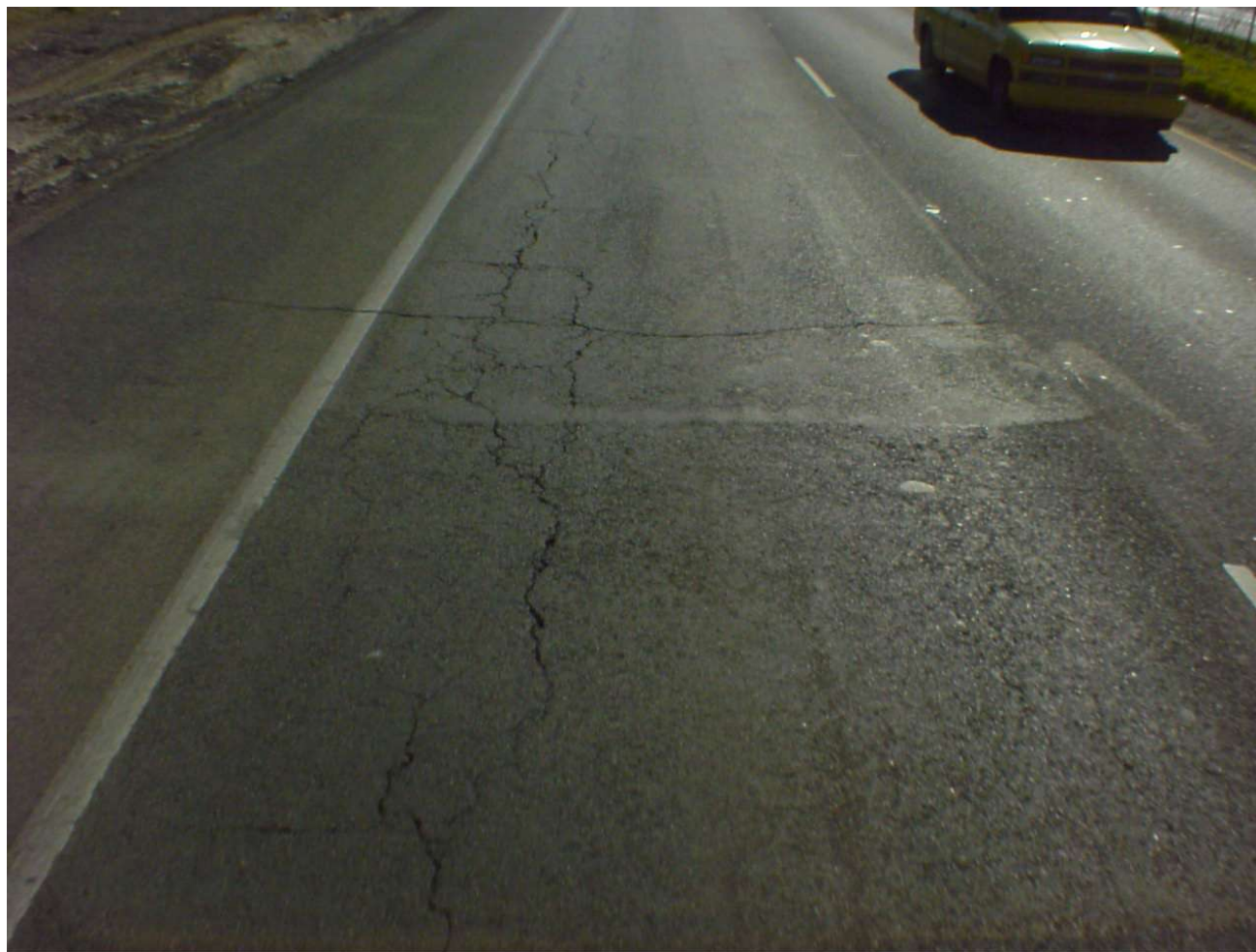
Figure 8-16: Example Distresses on SC Zone RAC Sections
