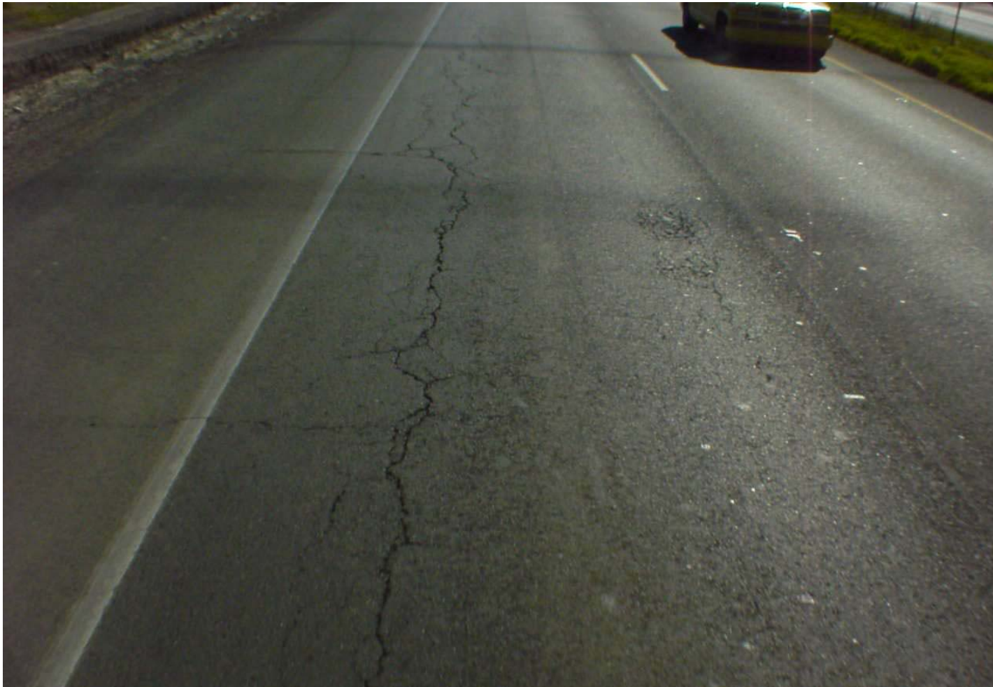
Figure 8-14: Example Distresses on SC Zone RAC Sections
