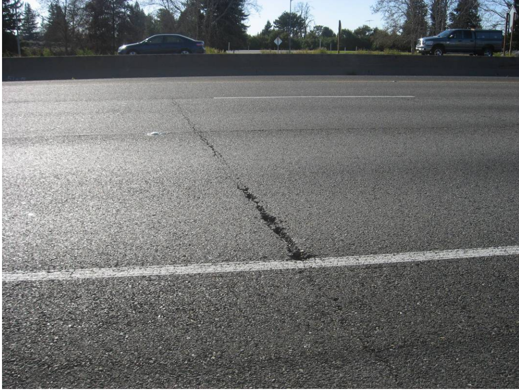
Figure A.14: Wide reflective cracks in the monitoring section in the NB direction.
