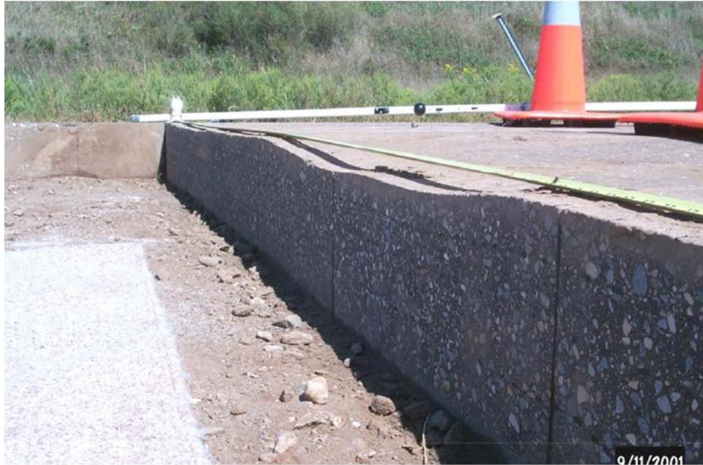
Figure 3.3: Photograph of the cross section of rutted HMA layer in trench in Cell 21 after trafficking.
