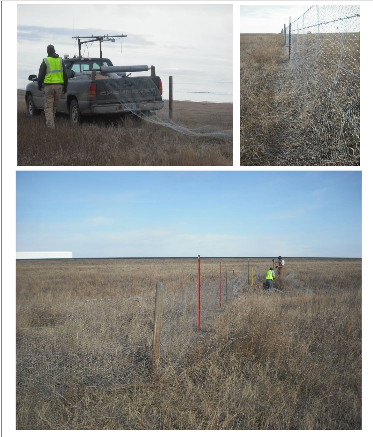
Figure 17. Fence installation (clockwise from top left: a vehicle-mounted spool aids in laying out ~5.6 km (3.5 mi) of fencing; several inches of mesh stapled to the ground creates a barrier to digging under the fence line; t-posts enable angling the mesh away from the right-of-way fence line (foreground) to the culvert entrances (location of workers in the mid-ground)).
