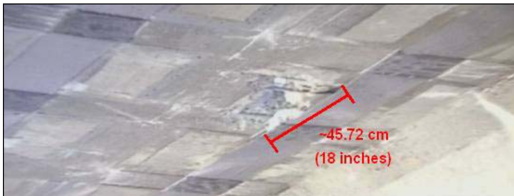
Figure 10.7. Punch Out of Bridge Deck in S9B5
