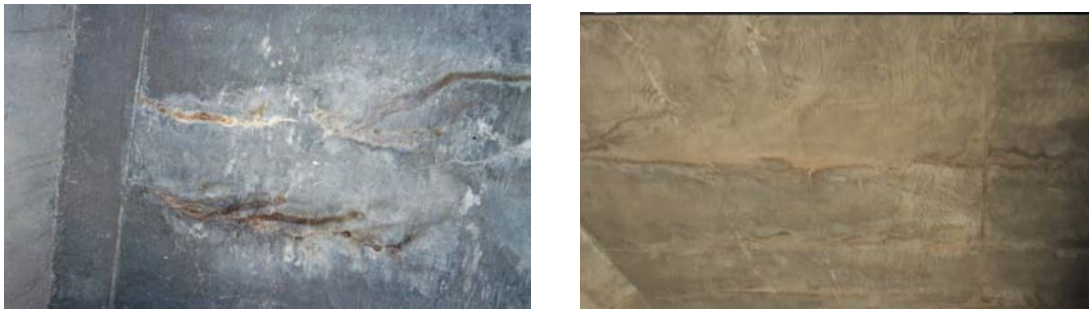
Figure 5.6. Transverse Cracking on Bridge Deck Soffit with Efflorescence
