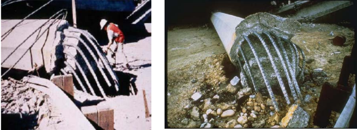
Figure 3.6: Column pull out failures during the San Fernando earthquake
