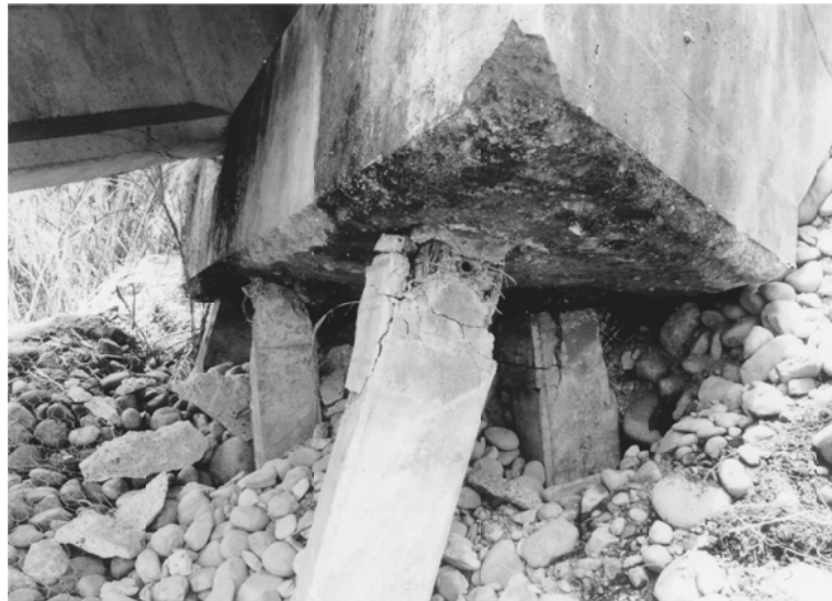
Figure 3.14: Abutment pile damage during the 1991 Costa Rica earthquake (Source: Moehle and Eberhard, 2003)
