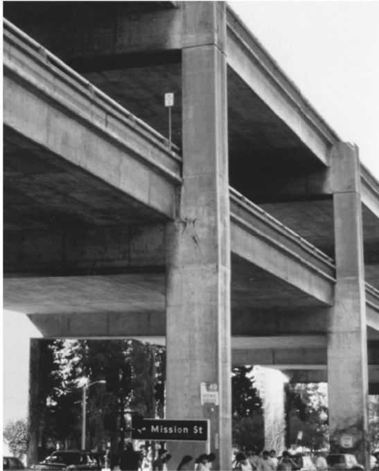
Figure 3.10: Joint damage to the Embarcadero viaduct during the Loma Prieta earthquake
