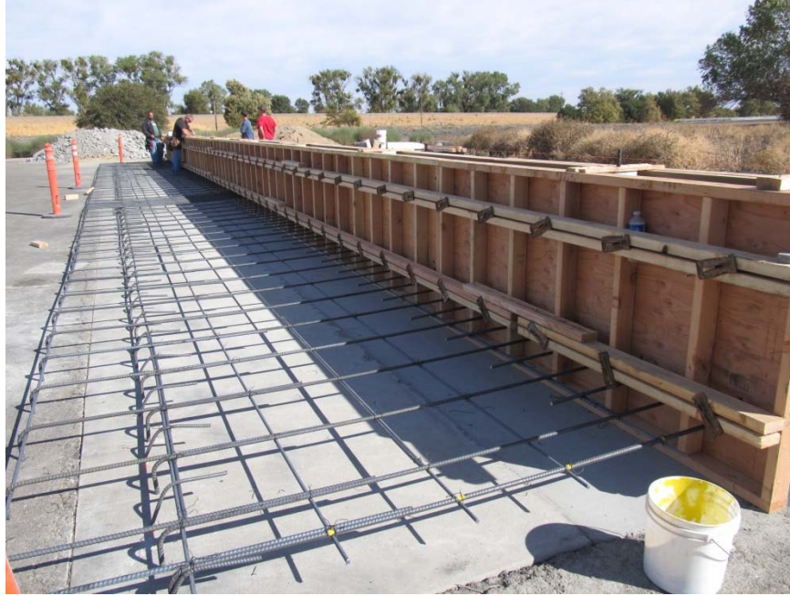
Figure 2-4 – Type 732SW formwork in place for the concrete parapet and rebar in place for the sidewalk
