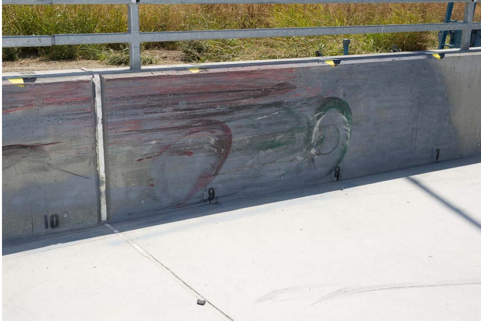
Figure 3-14 – Barrier face scraping after 130MASH3C13-02
