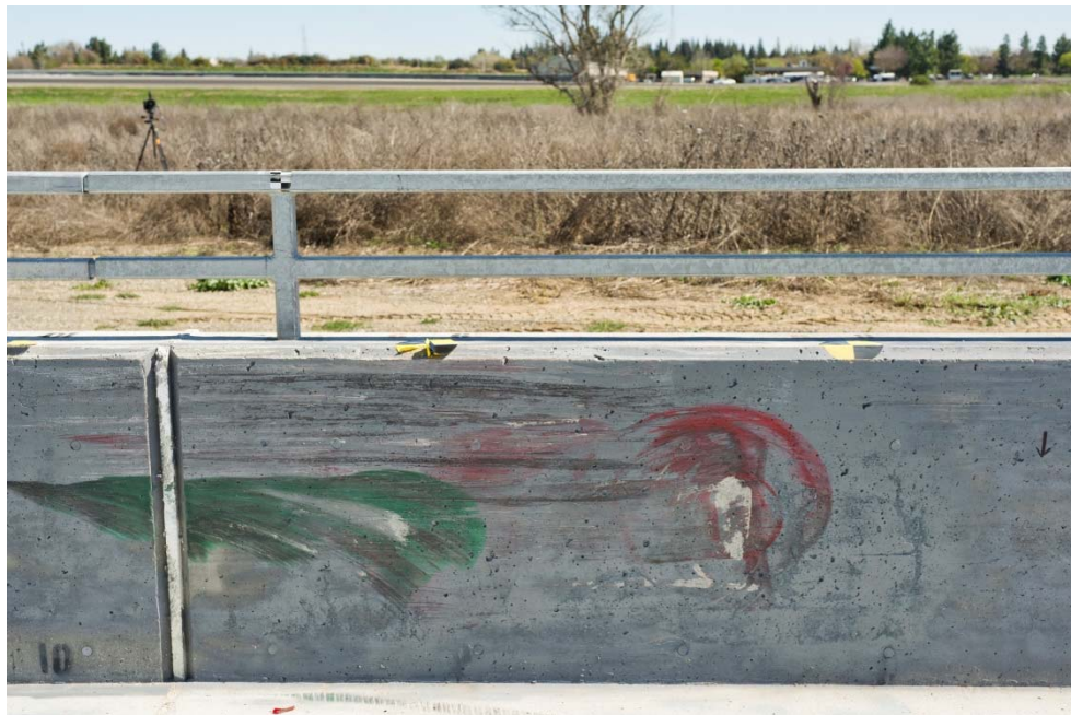
Figure 3-25 – 732SW Barrier face scraping after Test 110MASH2C14-01
