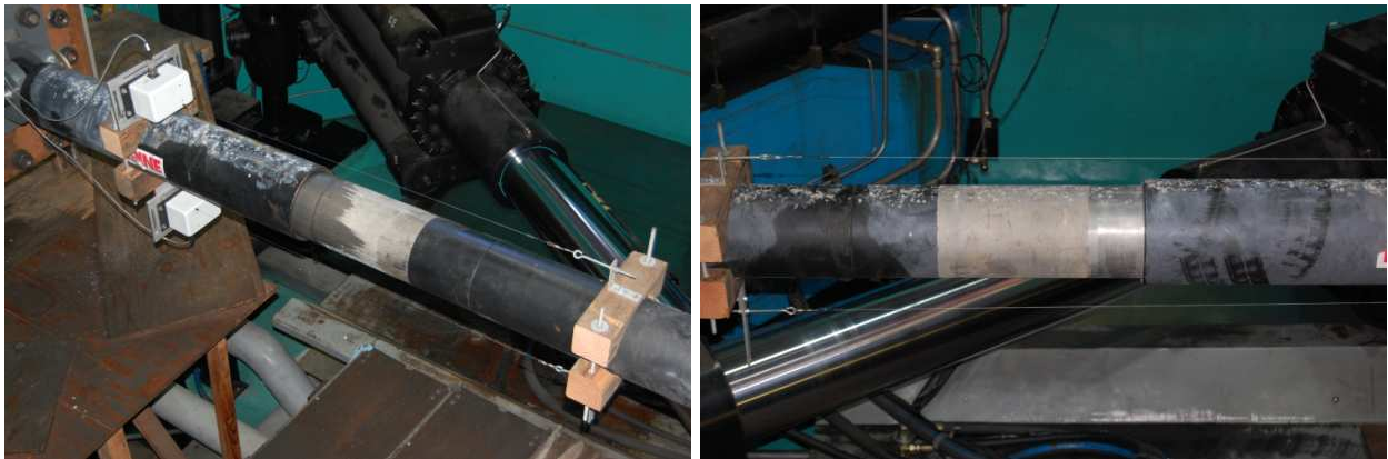
Figure 8 a) SN#006 leaking at the sleeve cover, b) SN#001 leaking at the threaded connection
